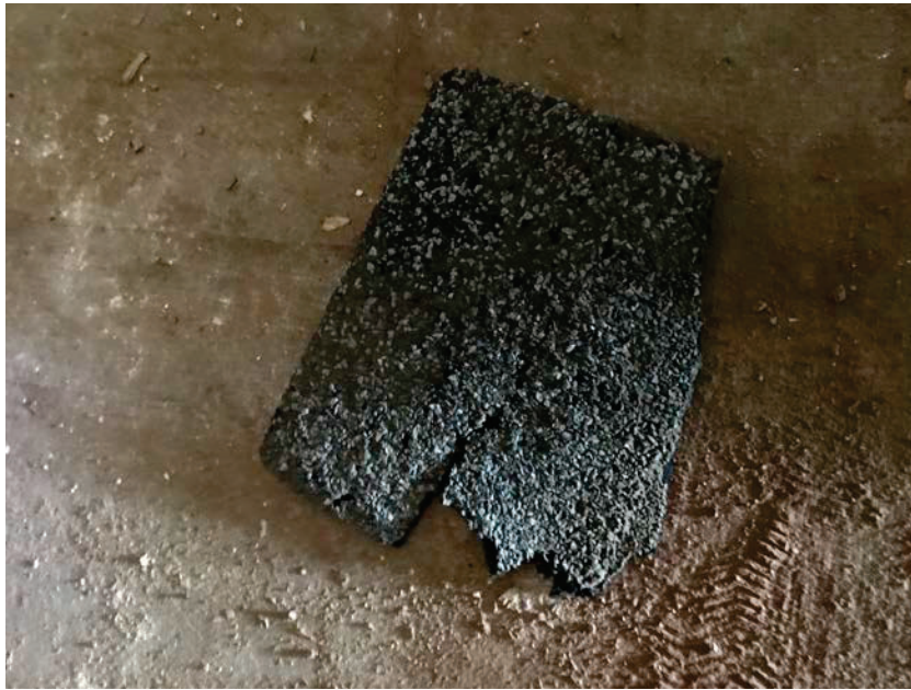
Photo 23: HA23 Roof shingles (B65-B67). Access to the roof was unavailable, roofing materials were collected in the attic near the roof access ladder.
