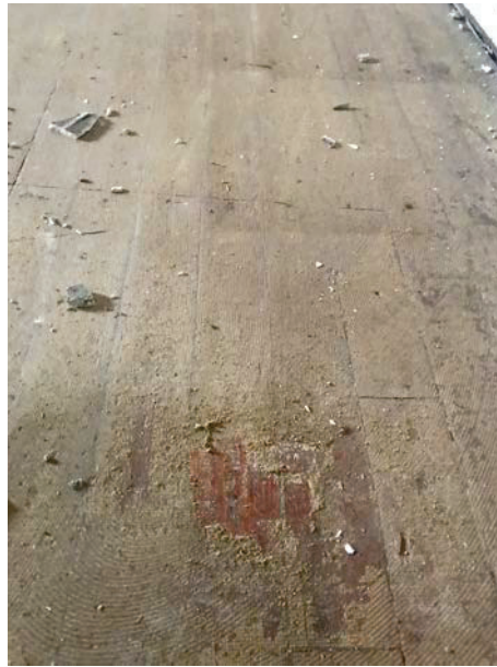
Photo 27: HA27 Residual yellow floor tile mastic on the 1 st floor (B77-B79)
