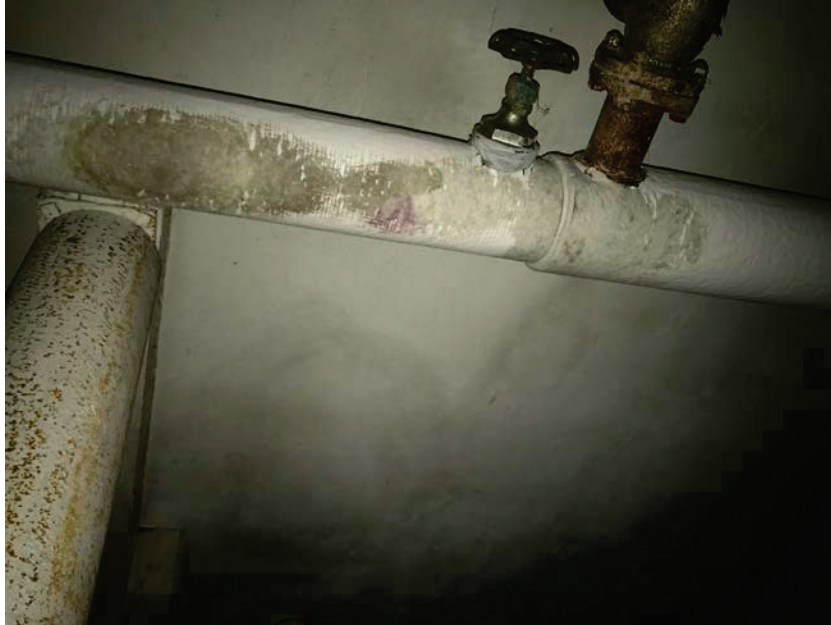
Photo 13: HA13 Pipe insulation on the pipes in the boiler room in the basement (B37-B39)
