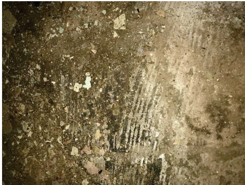
Photo 16: HA16 Residual black floor tile mastic in the corner of the rear right room of the basement, trace amounts (B45-B46)
