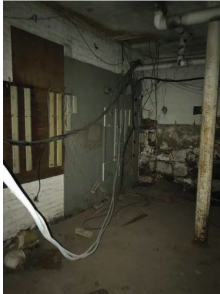
Photo 18: Wiring [Basement Boiler Room]
