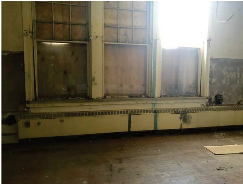
Photo 7: All single panel windows, window sills, window frames and window casing throughout the 1 st and 2 nd floor classrooms. Approximately 13 single panel windows throughout the 1 st and 2 nd floor classrooms.
