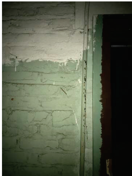
Photo 22: Brown and mint green paint on the wood door frame and door casing in the left side room of the basement right rear classroom. The mint green and white paint on the brick wall and metal pipes in the same room.
