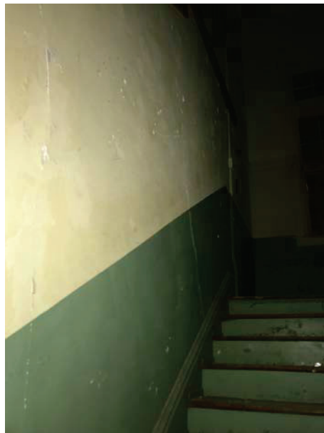
Photo 10: Green and cream paint on the plaster walls and wood stringer of the 1 st to 2 nd floor stairwell. Both sides of the stairwell.
