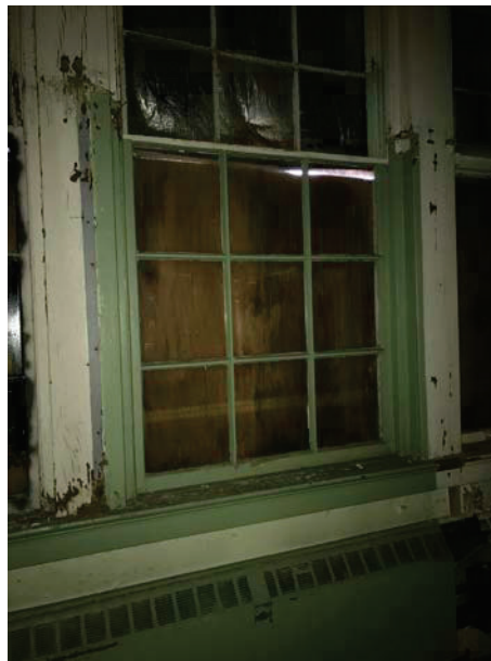
Photo 8: All multiple panel windows, window sills, window frames and window casing throughout the 1 st and 2 nd floor classrooms. Approximately 80 multiple panel windows throughout the 1 st and 2 nd floor classrooms.
