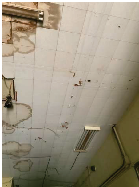
Photo 2: HA2 9"x9" white ceiling tiles with pinholes located in the 1 st floor hallway (B04-B06)
