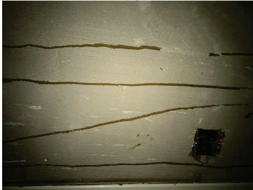
Photo 10: HA10 Tan wall glue lines on the walls of the 2 nd floor classrooms (B28-B30)
