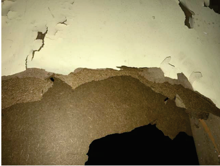
Photo 7: HA7 Brown felt paper in the walls in the 1 st floor hallway (B19-B21)
