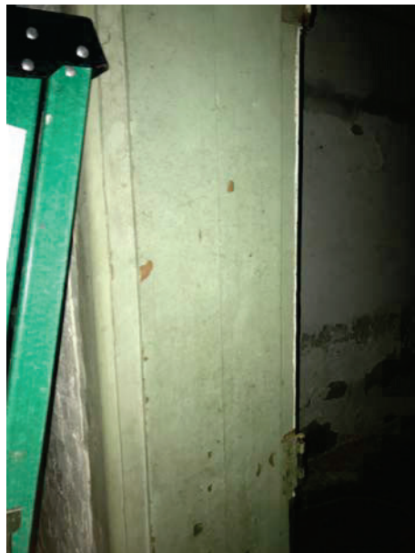
Photo 16: Green paint on the basement right front and left front classroom wood door casing.
