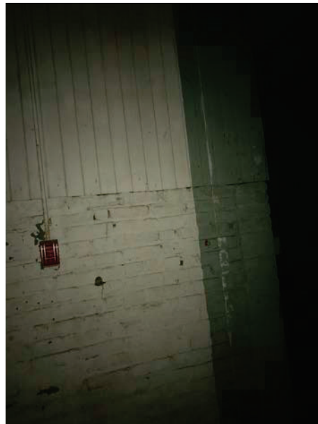
Photo 15: White and green paint on the wood paneling and brick wall of the basement stairs.
