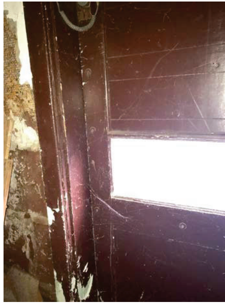
Photo 21: Brown paint on the wood door frame and door casing on the basement right exit door in the right rear classroom.
