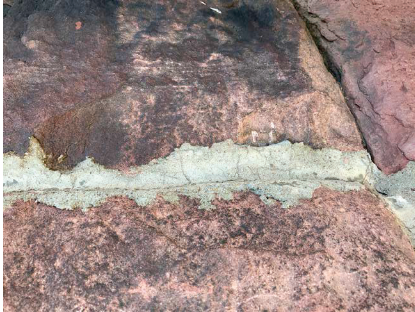
Photo 25: HA25 Gray brick mortar on the exterior of the subject property (B71-B73)
