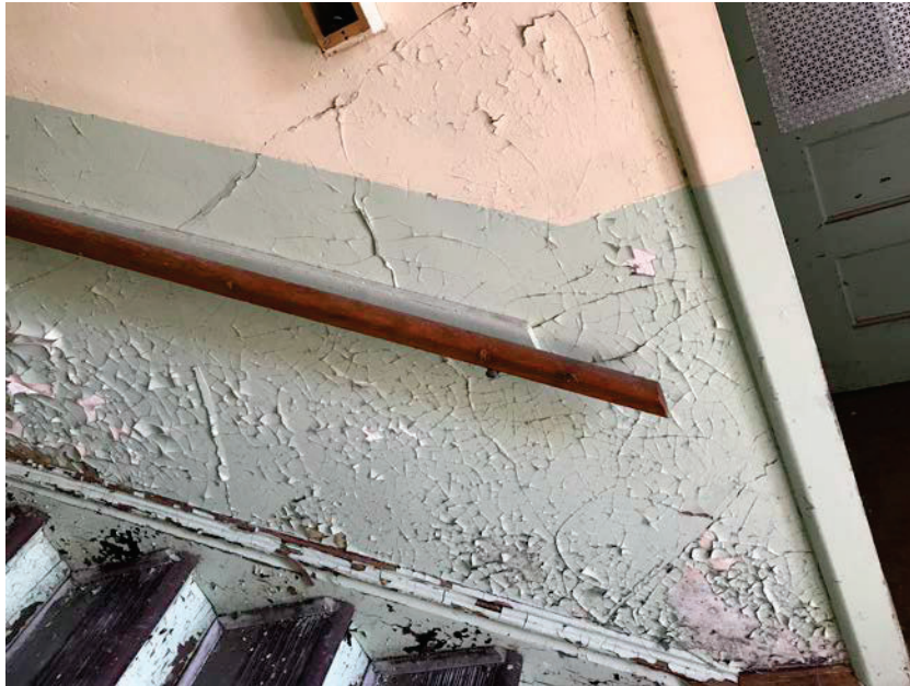
Photo 1: Mint green and cream paint on the plaster walls of the entrance stairwell. The mint green paint on the riser and stringer of the stairs. Both sides of the stairwell.
