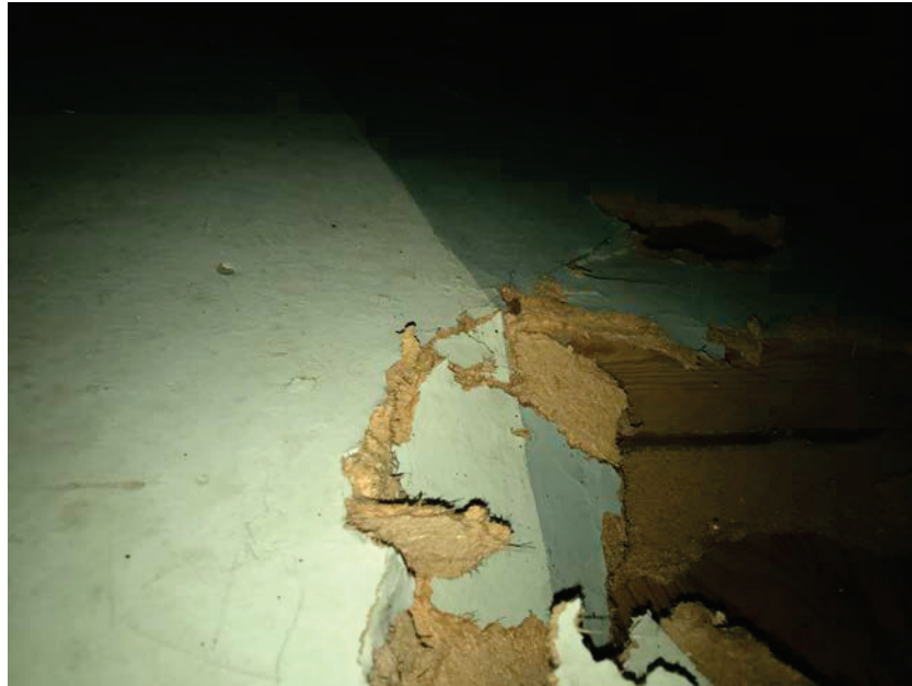
Photo 15: HA15 Brown drywall in basement classrooms (B42-B44)
