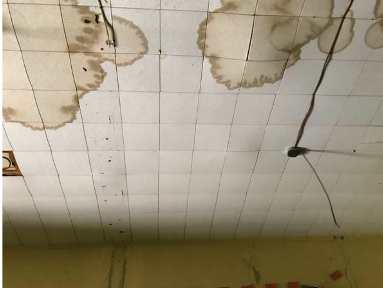
Photo 24: Water-Stained Ceiling Tiles [1 st Floor]
