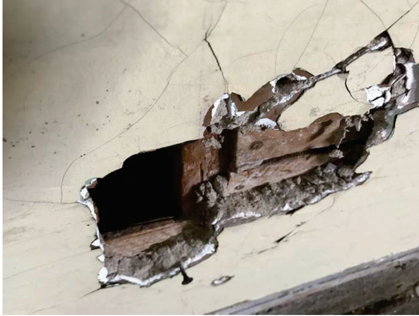
Photo 1: HA1 Plaster located throughout the subject property (B01-B03)
