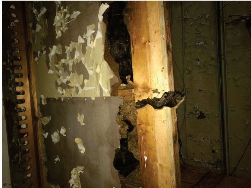
Photo 21: HA21 Brown insulation in the walls of the 1 st floor hallway (B59-B61)
