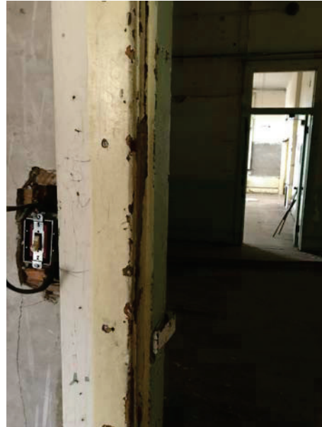
Photo 4: Mint green paint on the wood door casing in the left rear classroom on the 1 st floor. Cream paint on the door frame in the left rear classroom on the 1 st floor.
