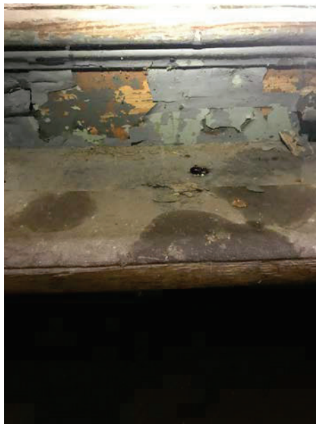
Photo 14: Blue gray paint on the basement stair risers on both sides.
