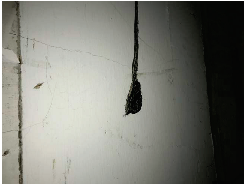
Photo 11: HA11 Black wall glue lines on the walls of the 2 nd floor classrooms (B31-B33) 3% Chrysotile
