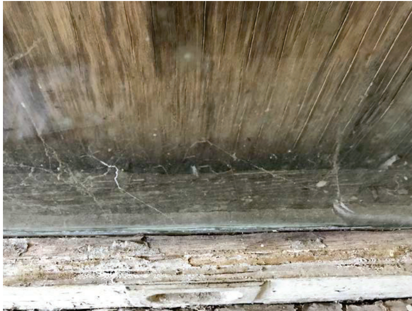
Photo 20: HA20 Exterior window caulking on the single panel windows of the subject property (B56-B58)
