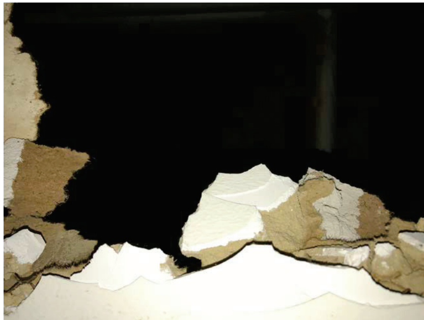
Photo 4: HA4 Joint Compound located throughout the subject property (B10-B12)
