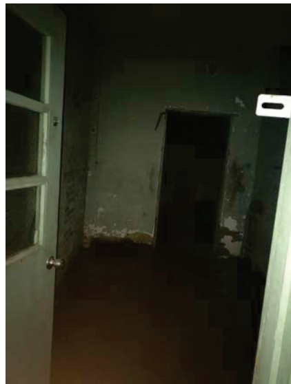
Photo 20: Mint green paint on the walls, door, door frame and door casing in the basement left rear entry room to the left rear classroom.
