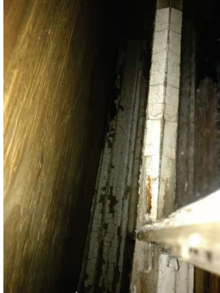
Photo 6: HA6 Exterior window glazing on the multiple panel windows throughout the subject property (B16-B18)
