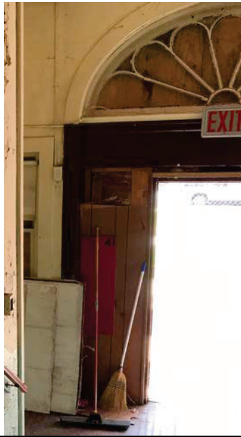
Photo 9: HA9 Caulking on the window boards covering the exterior windows of the subject property. The sample was collected from an extra window board at the front entrance (B25-B27)
