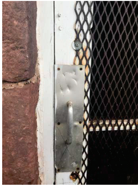
Photo 25: White paint on the exterior right exit door
