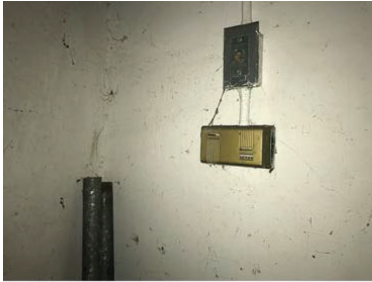
Photo 17: Thermostat [Corner of Northeastern basement room]
