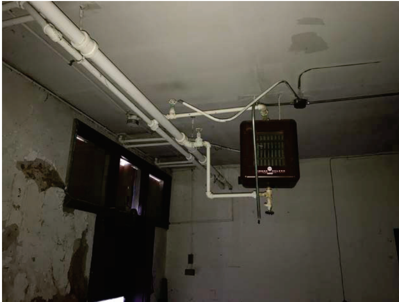
Photo 15: Unit Heaters [multiple in basement]
