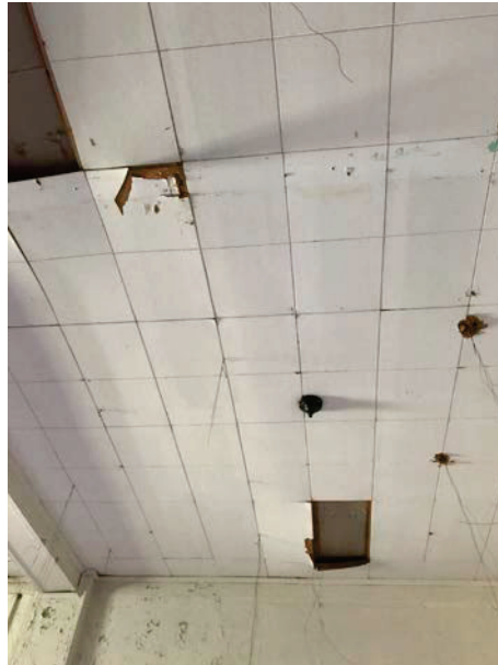
Photo 5: HA5 14"x14" white ceiling tiles located in the classrooms throughout the subject property (B13-B15)
