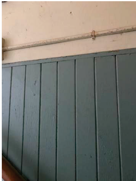
Photo 13: White paint on the brick the basement stairwell on both sides. White drywall overhang in this area on both sides of the basement stairs.
