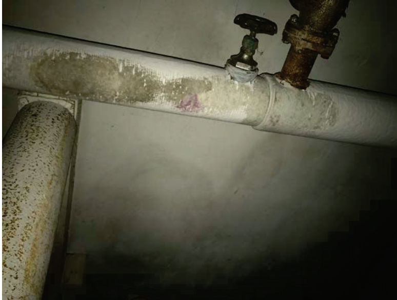
Photo 20: Boiler Pipe Insulation [Basement Boiler Room]
