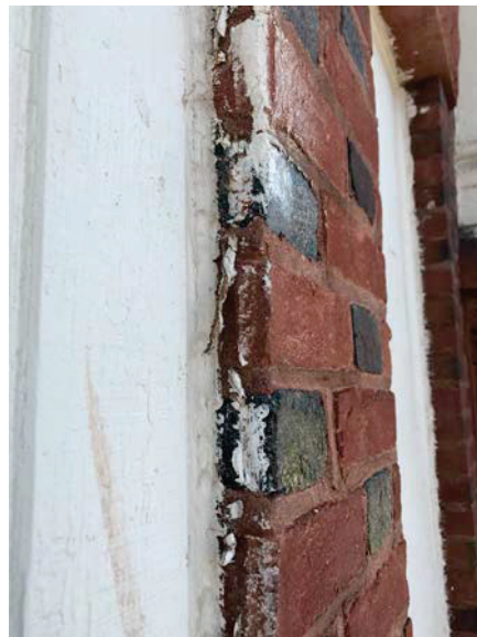
Photo 26: HA26 Exterior front door caulking (B74-B76) 5% Chrysotile
