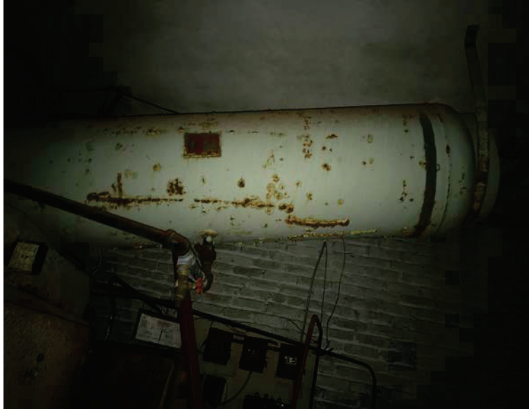
Photo 19: Boiler Tanks [Basement Boiler Room]
