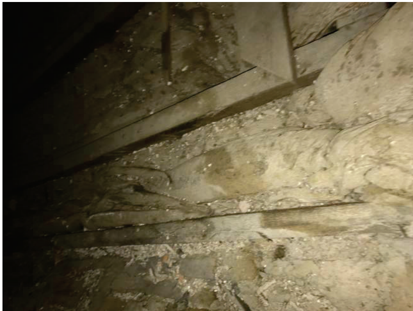
Photo 24: HA24 Attic insulation (B68-B70)
