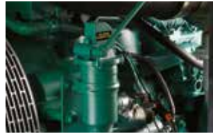
Lube oil drain pump
