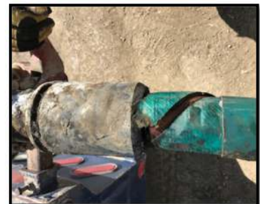
Figure 3.0 – Failure by High-Rate Back-Flow from Injection Wells
