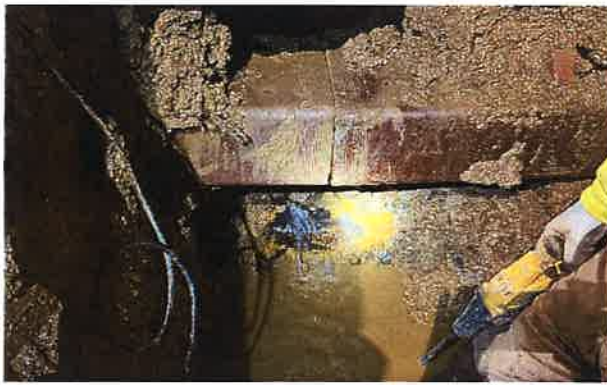
Main Break – Ferris Street @ S. Main Street
