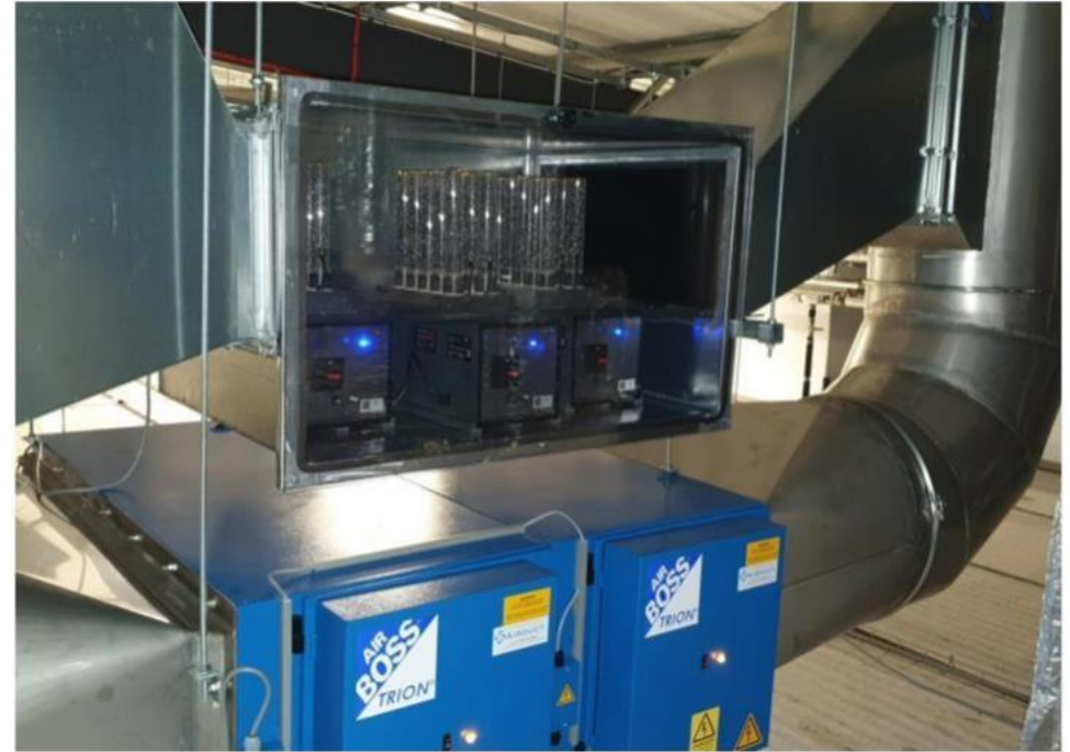
Kitchen exhaust unit
