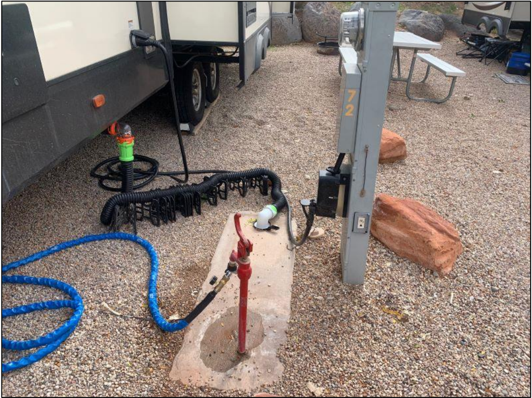
Water, Sewer/Waste, Power Hookups
