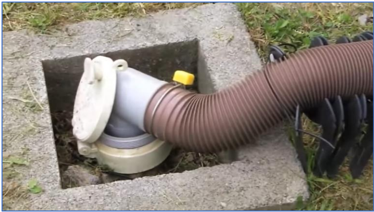
Residential sewer clean-out with RV waste Line connection
