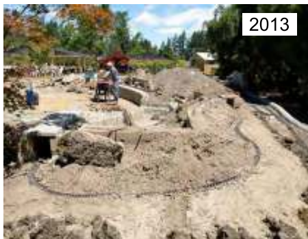
Layout #3 early in construction in 2013; concrete blocks in place with fill dirt being added.
