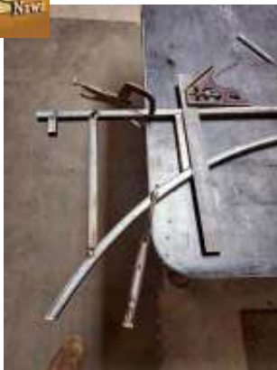
Photo 5 Using a carpenter's square to line everything up. Note the tack welds.
