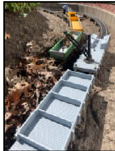
Workers finally reached the tunnel portal, but opening the secure tunnel door will not be for a few weeks.
