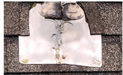
Damaged or aged roof jacks may allow water leaks in your roof.
