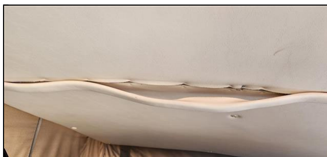
Ceiling Seam Coming Apart
