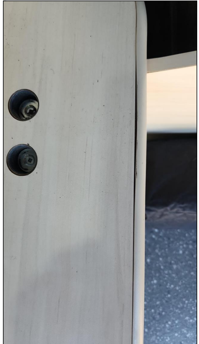
Trim on Cabinet by Back Door
