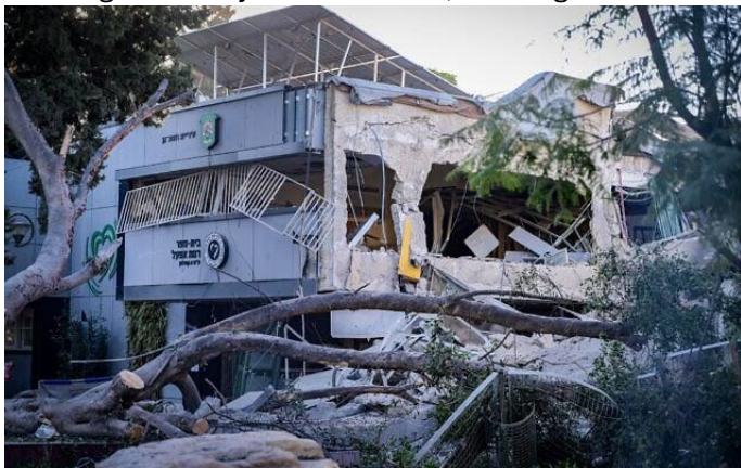
The damage caused from a ballistic missile fired from Yemen, at a school in Ramat Gan, December 19, 2024. (Avshalom Sassoni/Flash90)
