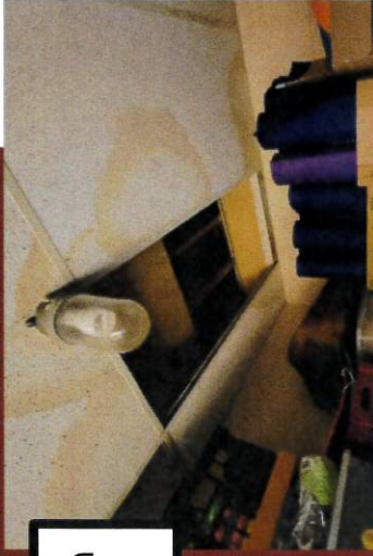
Water damage from poor roof design
