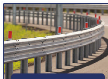
Metal Beam Crash Barrier
