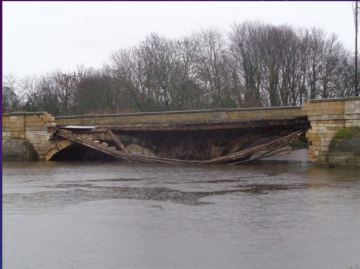
Partially collapsed Tadcaster Bridge (30th December 2015) The bridge on the day after the collapse. This collapse also caused a substantial gas leak
