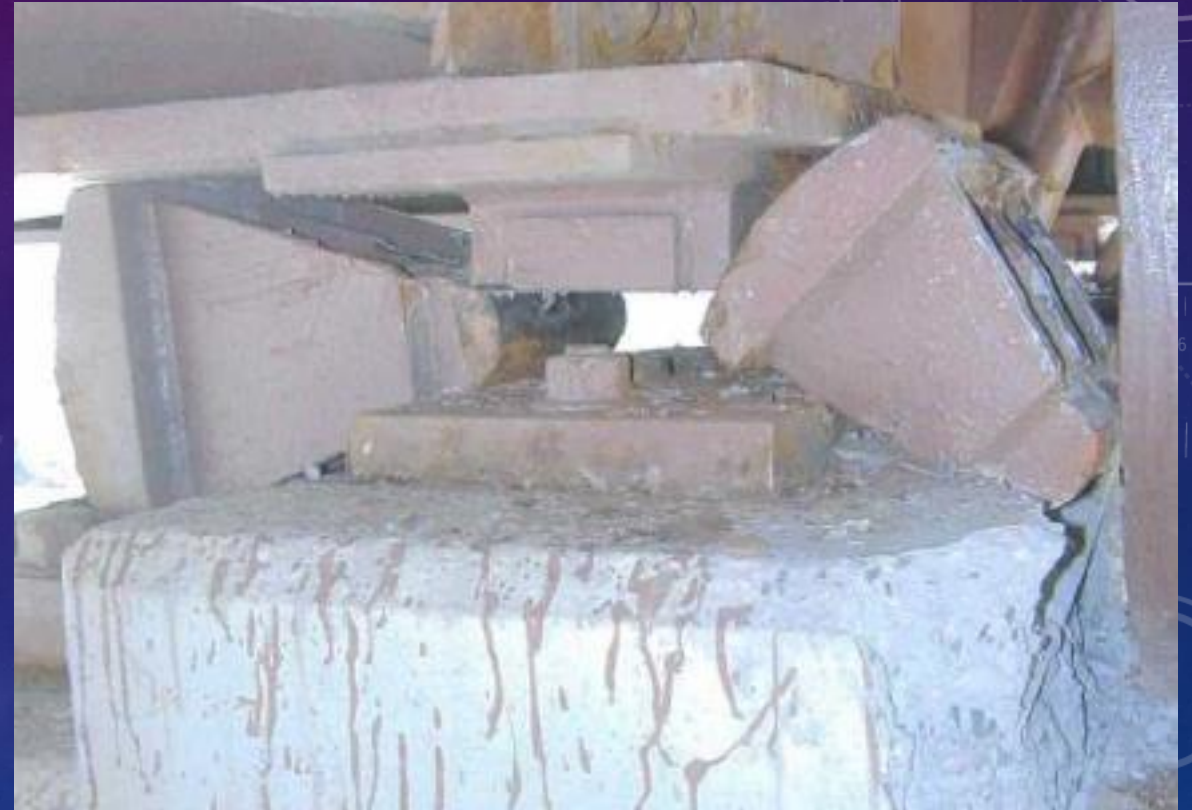
Failed Condition at East Fascia
