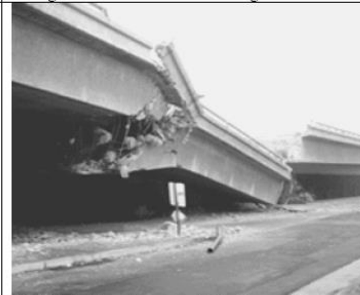
1994 Northridge – Interstate 10, La Cienega Bl. Column failure, bridge collapse
