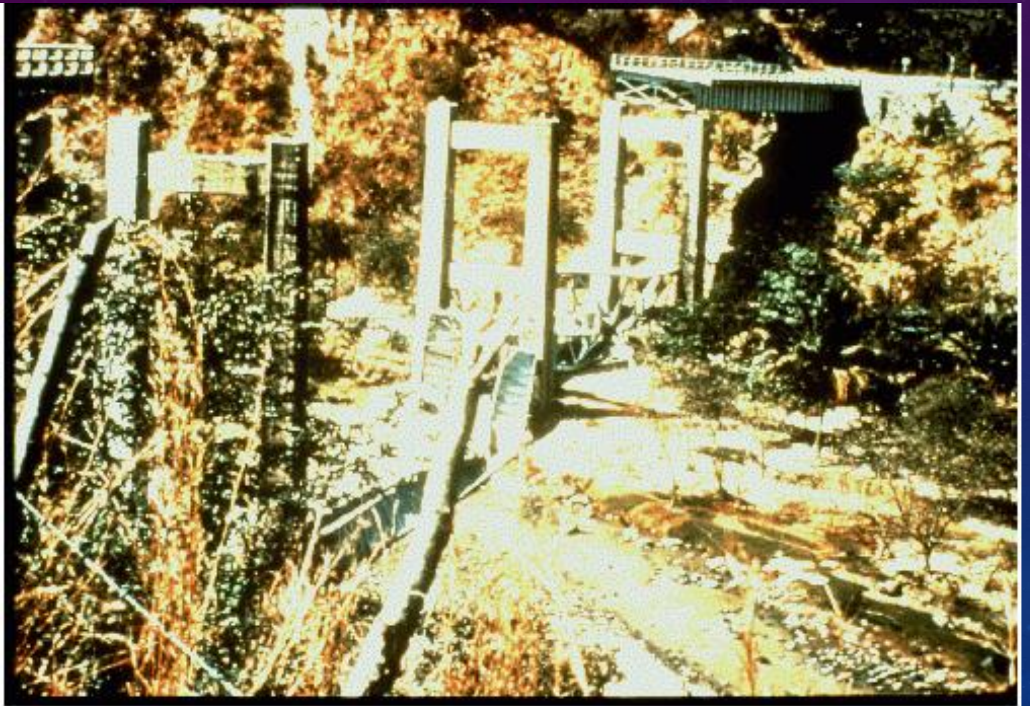
Collapse of Spans on Bridge Due to 1976 Earthquake in Guatemala
