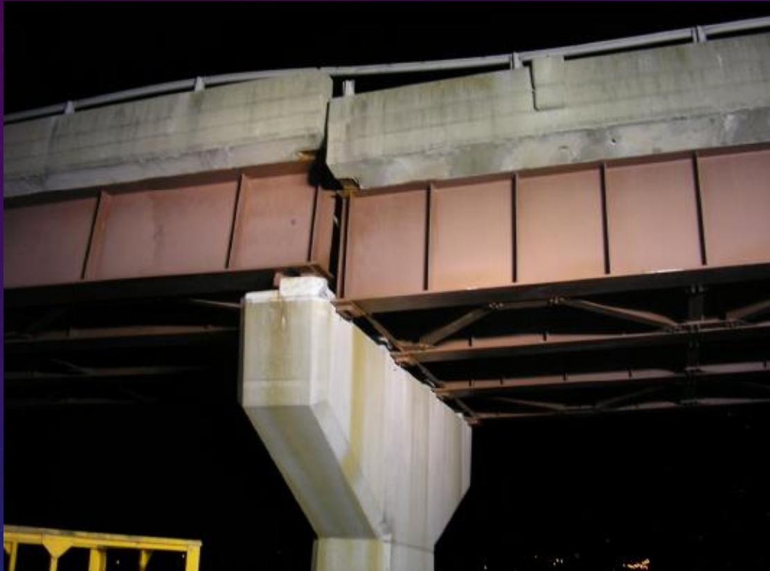
Partial Failure Pier 11, East Fascia
