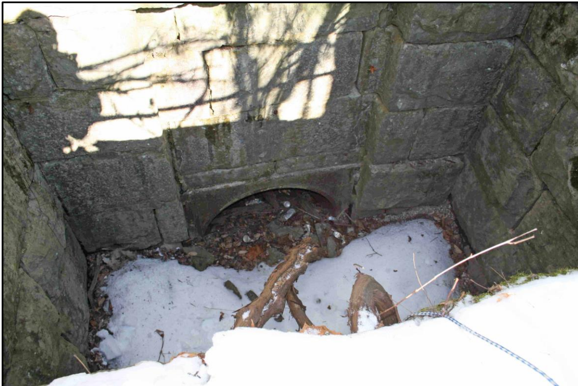
Figure 9 (top) and Figure 10 (bottom). 2015 views of the Owasco Feeder bulkhead (courtesy of Mike Riley).
