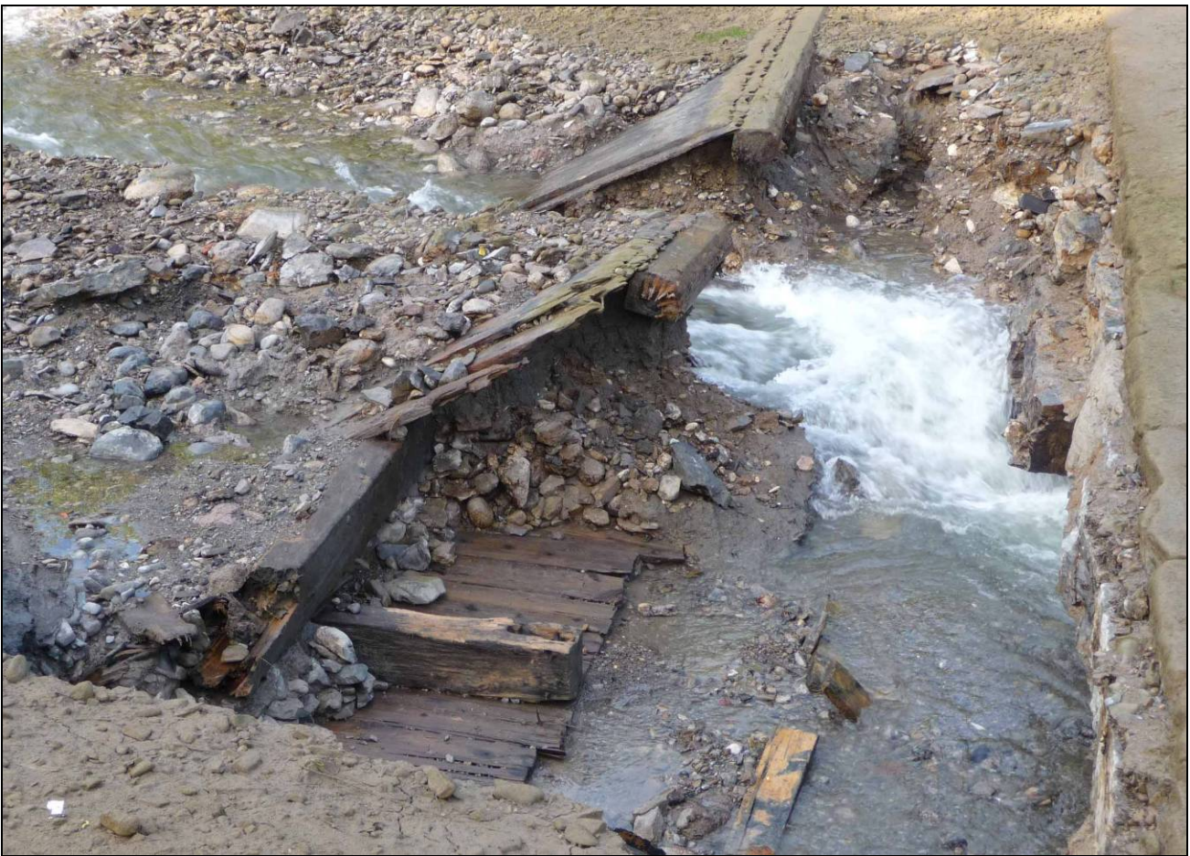
Figures 21, 22 and 23. Failure of the Limestone Creek Feeder Dam in 2009 (Village of Fayetteville).
