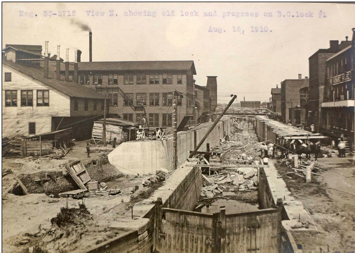
Figure 64 (top). View north over Enlarged Oswego Canal Guard Lock 1 in Phoenix, c1905; Figure 65 (bottom). View north over construction of Oswego Barge Canal Lock 1 with Guard Lock 1 in foreground, August 16, 1910.
