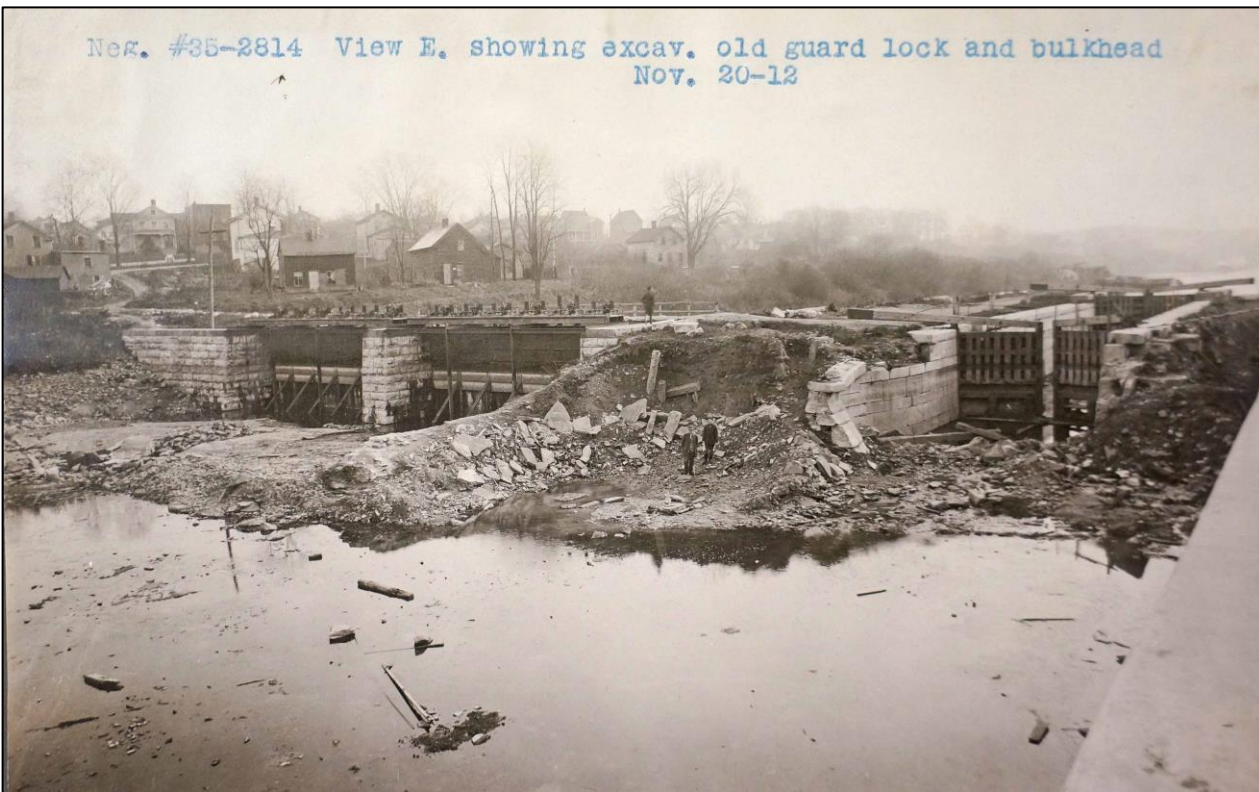
Figure 42 (top). View south towards Enlarged Oswego Canal Guard Lock 5 (right) and the bulkhead to the Oswego power canal (left) with the corner of the Weighlock pier on the far right, October 17, 1907; Figure 43 (bottom). View southeast over the guard lock and power canal bulkhead, November 20, 1912.
