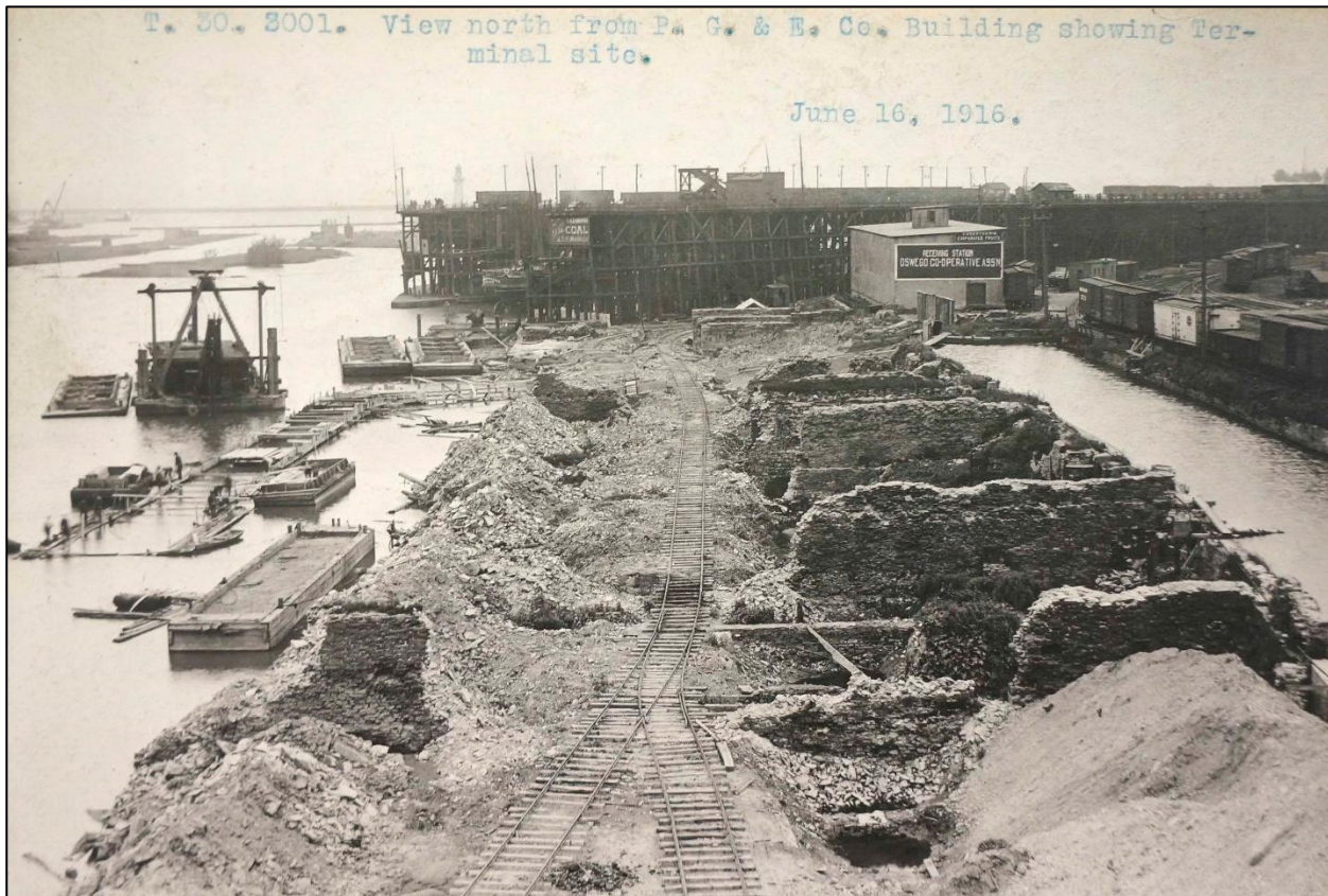
Figure 16 (top). View from top of grain elevator looking south down First Street, May 18, 1925; Figure 17 (bottom). Preparing the site for the State's Barge Canal Terminal at Oswego, looking north, June 16, 1916.
