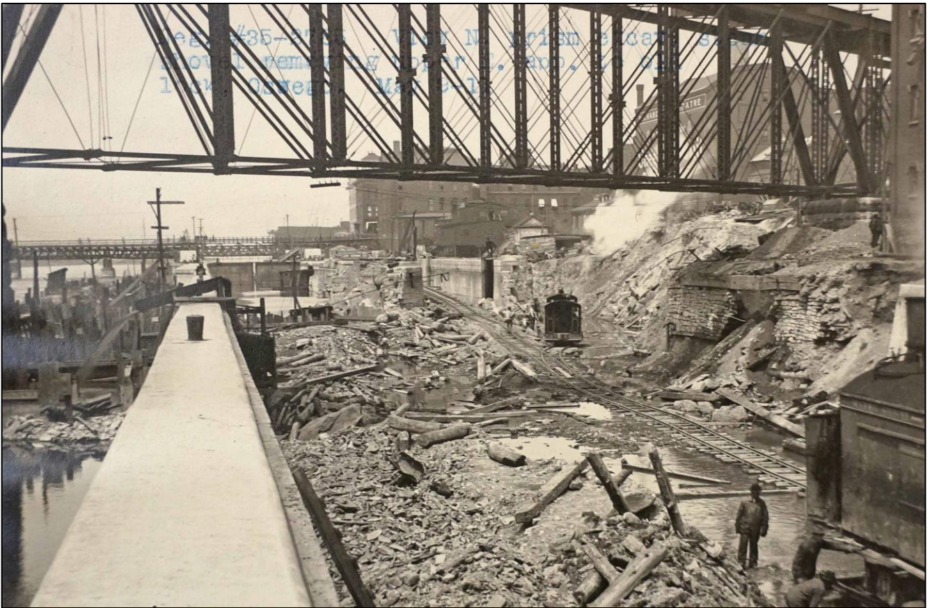
Figure 25 (top left). View north down the Oswego River with Enlarged Oswego Canal Lock 18 on right, c1905; Figure 26 (top right). View north down the Oswego power canal on right with Lock 18 on left; Figure 27 (bottom). View north down the channel of the Barge Canal with Oswego Barge Canal Lock 8 in the distance on left and Enlarged Oswego Canal Lift Lock 18 on right.
