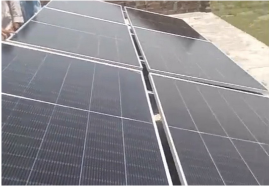
Solar power installed for the ministry facility
