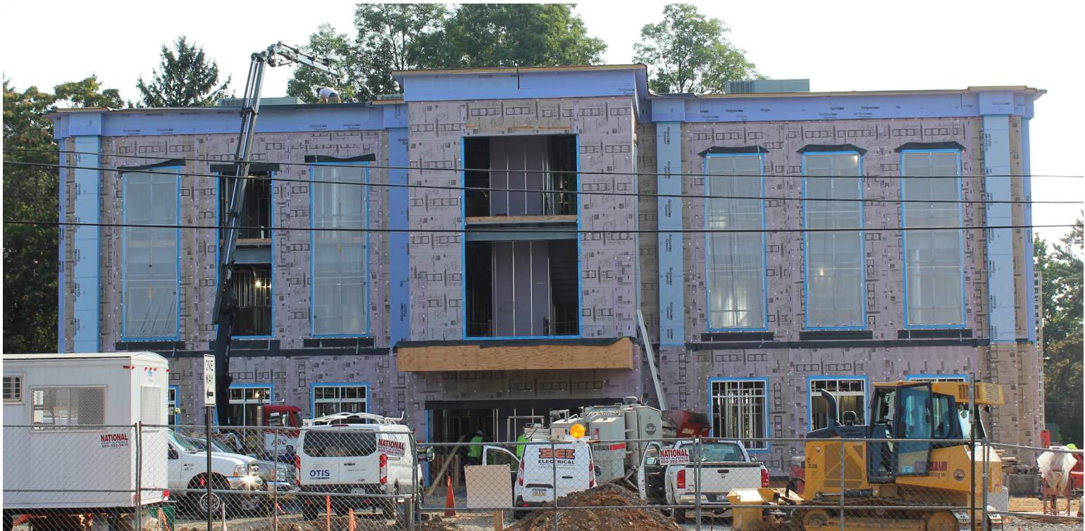
Medical offices at 834 Eaton Avenue in Bethlehem City, Photo by Craig Kackenmeister/LVPC
