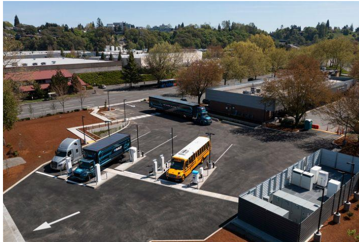
Figure 28: Heavy-Duty Electric Charging Station in Portland, OR
