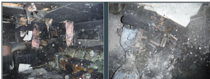
LITHIUM-ION BATTERY FIRE / Hoverboard
