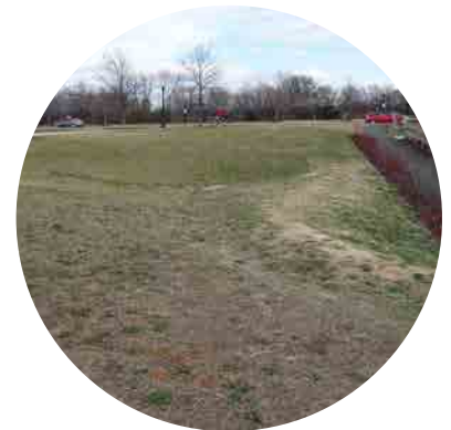
STORMWATER INLET GRATE
