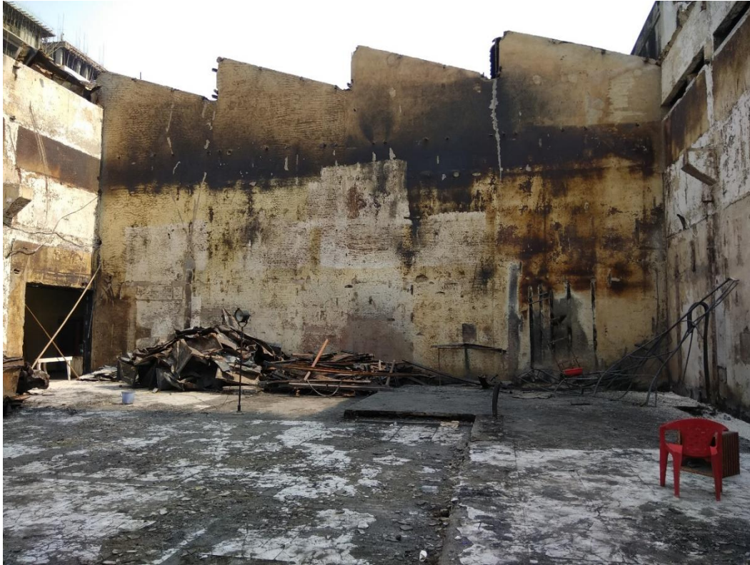
Figure 1 Fire Damaged Structure
