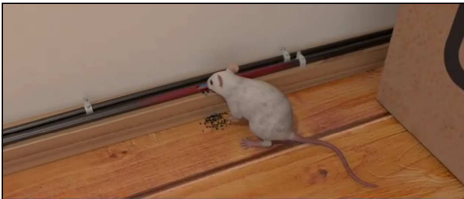
Pets or rodents can damage cables
