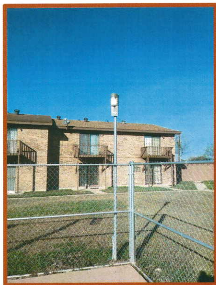
Swimming Pool Lights / Light Poles
