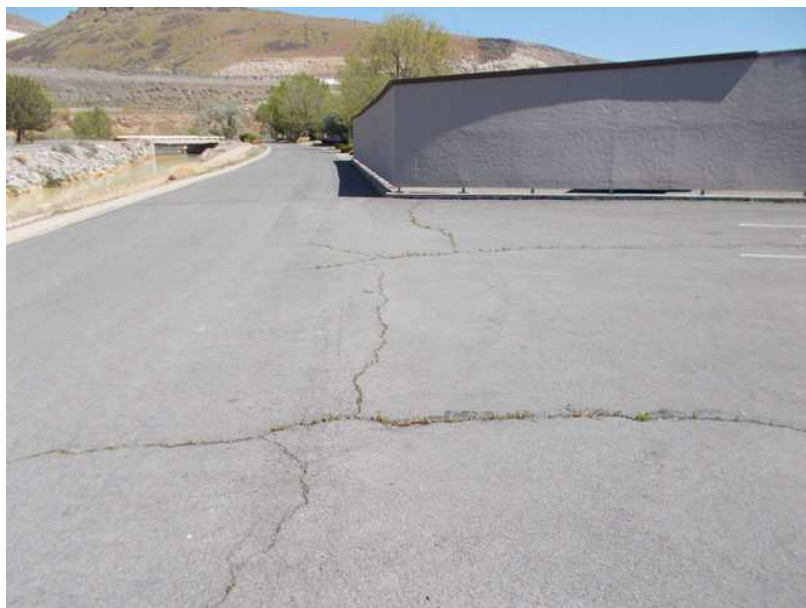
The Asphalt Road Maintenance Schedule includes the Surface Maintenance Treatment, Overlay and Crack Seal. This Schedule is an estimation only.
