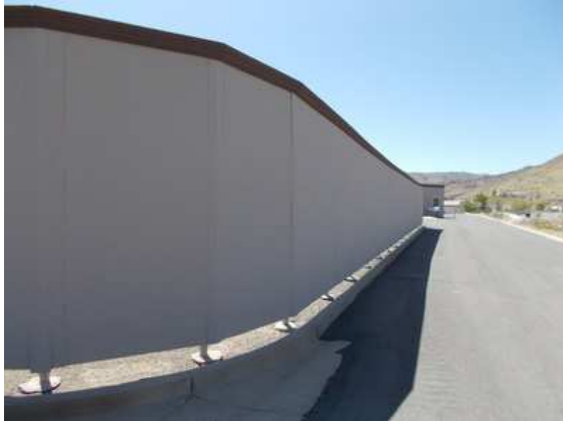
Repair and Painting of the Wooden Fencing around the Lot A & B Parking Area has been included in the Study.
