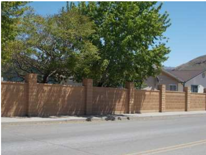
Perimeter Wall Repairs have been included in the Study as an allowance, to be done as needed.
