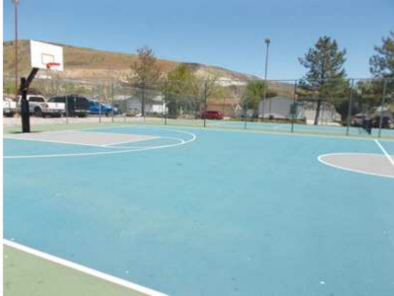
The Tennis Court Resurface, Sealing, Basketball Hoops and Chain Link Fencing have been included in the Common Area Category.
