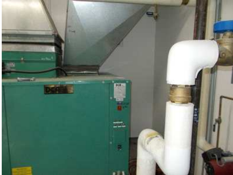
The Estimated Useful Life and Replacement Costs of the De-Humidifier/ Ventilation System and Pool Equipment was provided by Lee Joseph Pools, Reno, Nevada.
