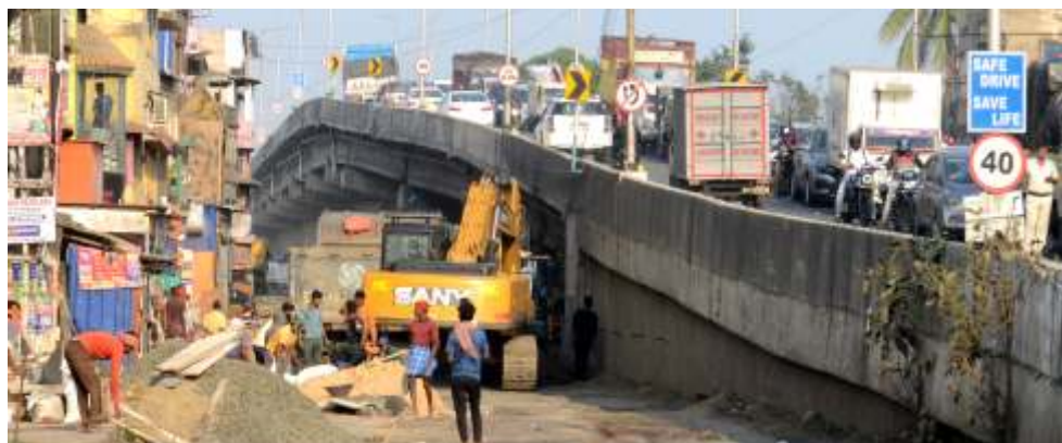
PWD workers are busy in improvement & strengthening work of the Budge Budge Trunk Road beside Sampri Flyover near Bata More. It is a Govt of West Bengal project under PWD, South 24 Pargans Division. (Pic: Debajyoti Sarkar)
