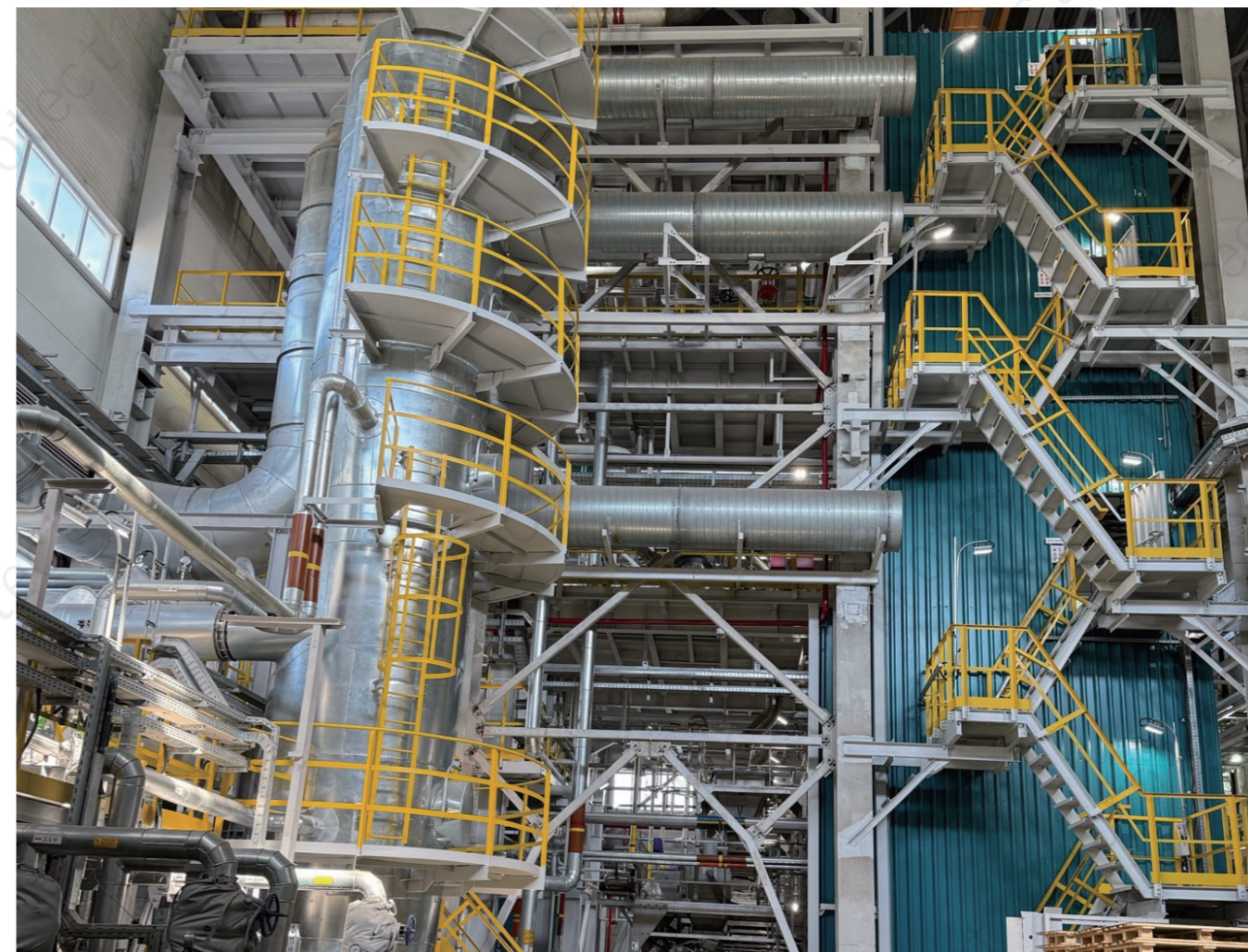
Scrubber Systems for Chemical and Maleic-Anhydride Service
