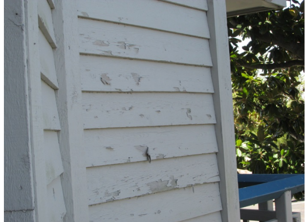
Paint finish deterioration
