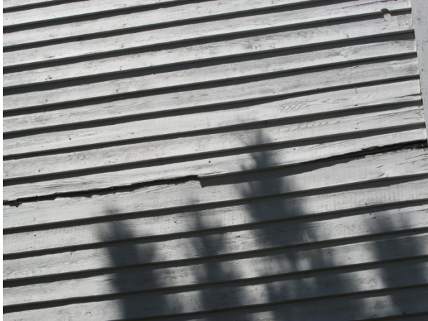
Wood siding deterioration
