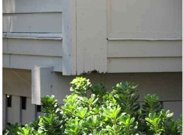
Wood trim deterioration
