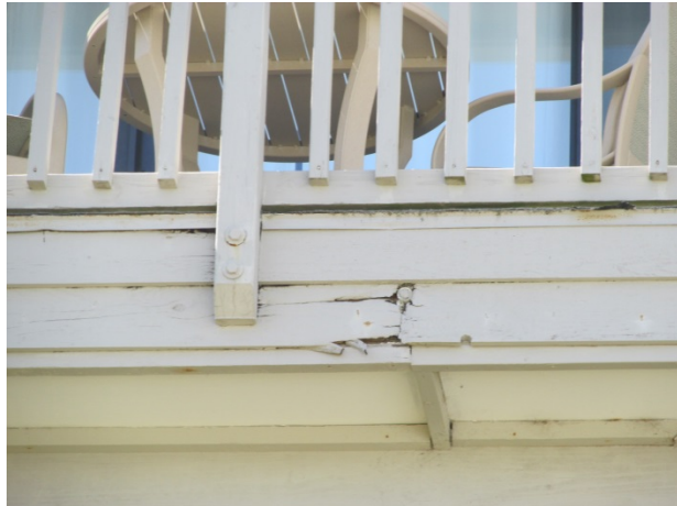
Isolated fascia deterioration at the balconies
