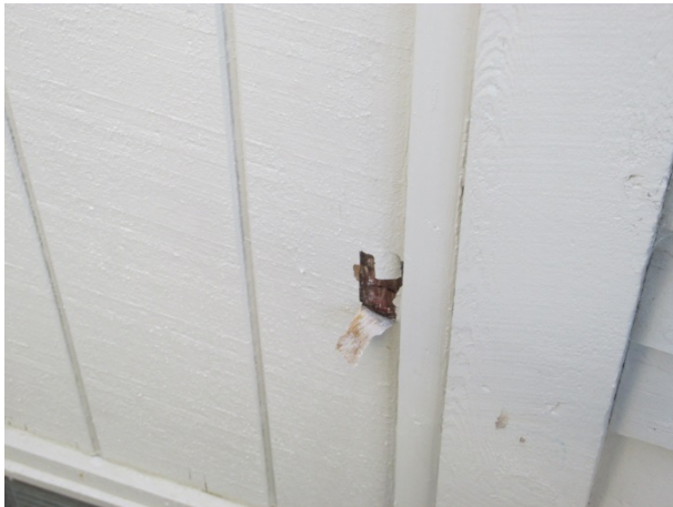
Paint finish deterioration
