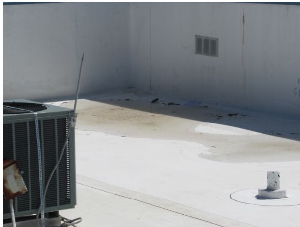
Standing water at the roof
