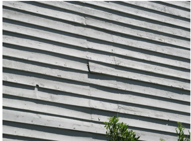
Wood siding deterioration
