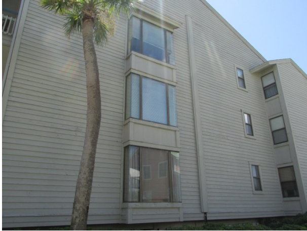
Paint finishes in fair- to poor-condition
