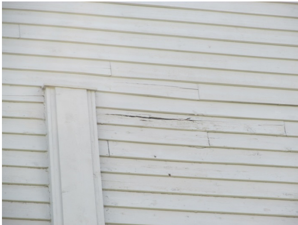
Wood siding deterioration
