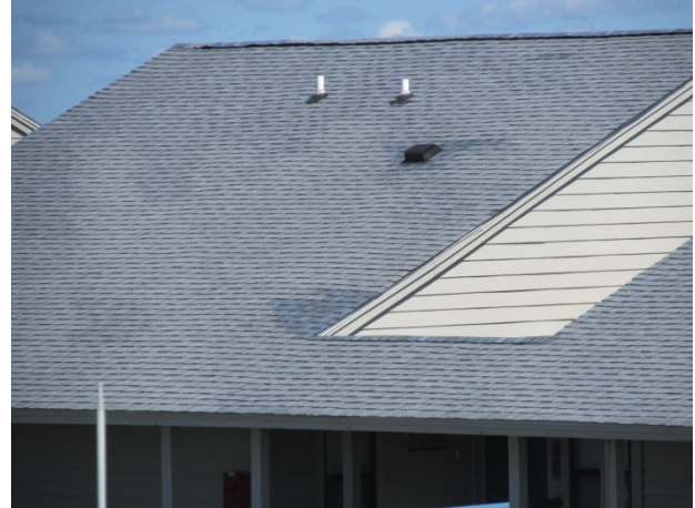
Isolated replaced sections of shingles
