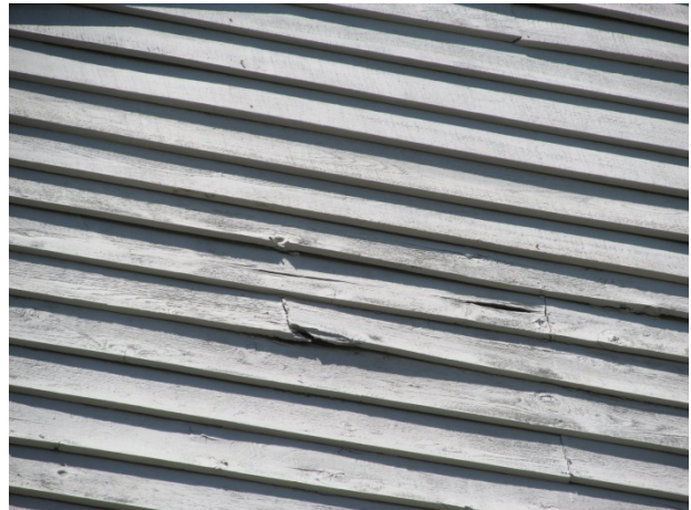
Wood siding deterioration
