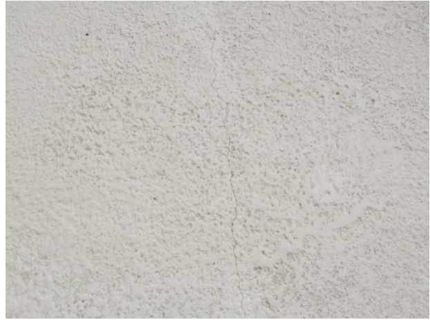
Isolated crack at the deck
