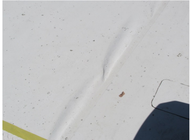
Isolated bulges at the roof
