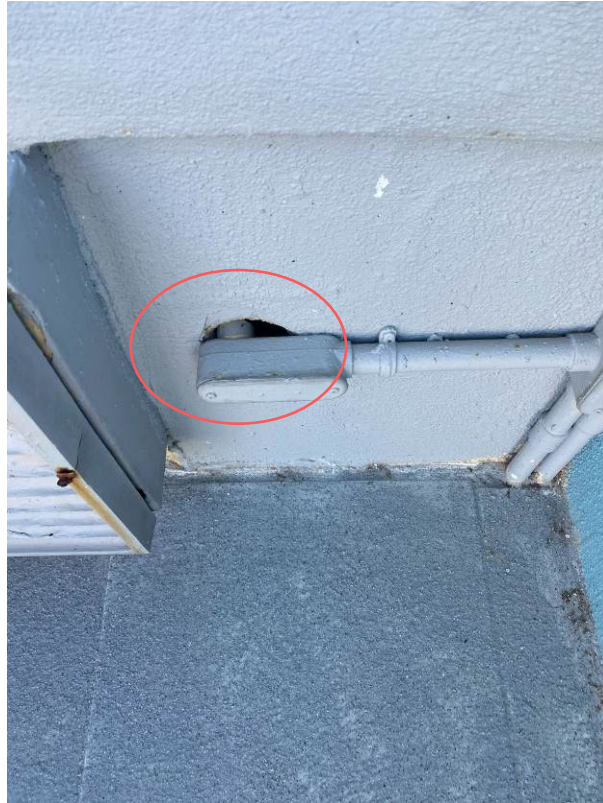
Photograph #29 – Typical unsealed hole at electric penetration
