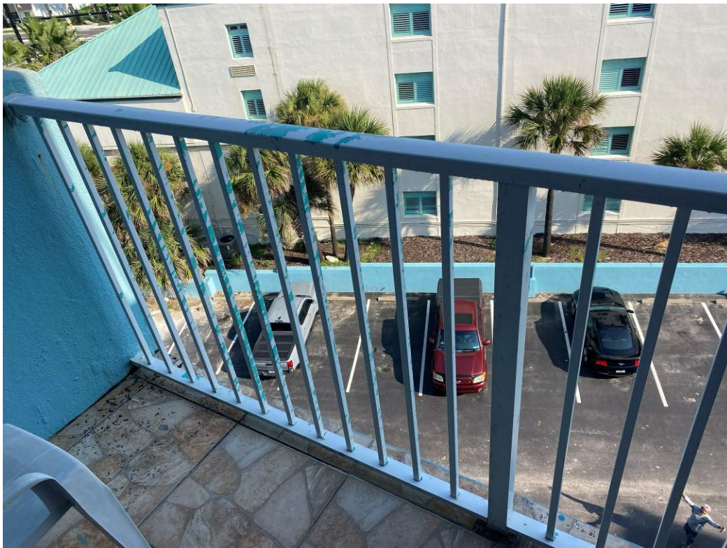
Photograph #30 – Typical paint peeling on guardrail
