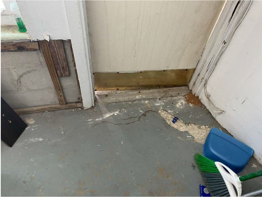
Photograph #7 – Typical interior topside concrete spall
