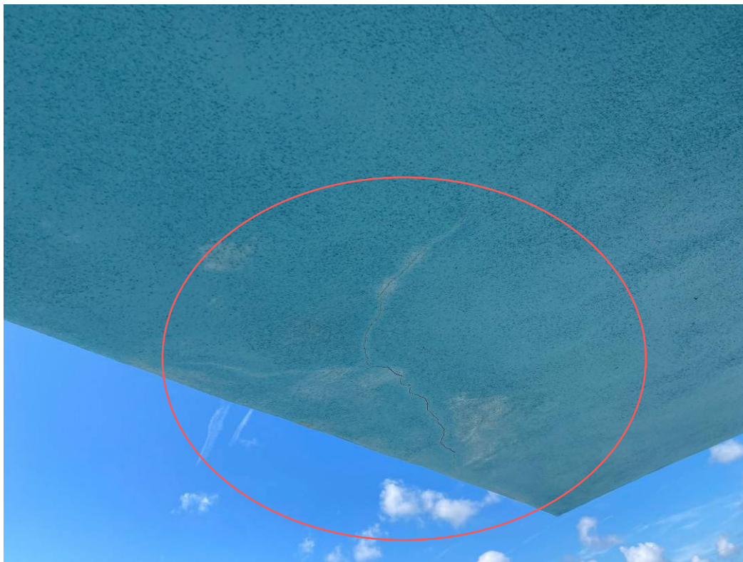
Photograph #20 – Typical ceiling spalling
