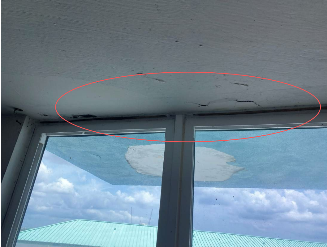
Photograph #13 – Typical interior ceiling spalling
