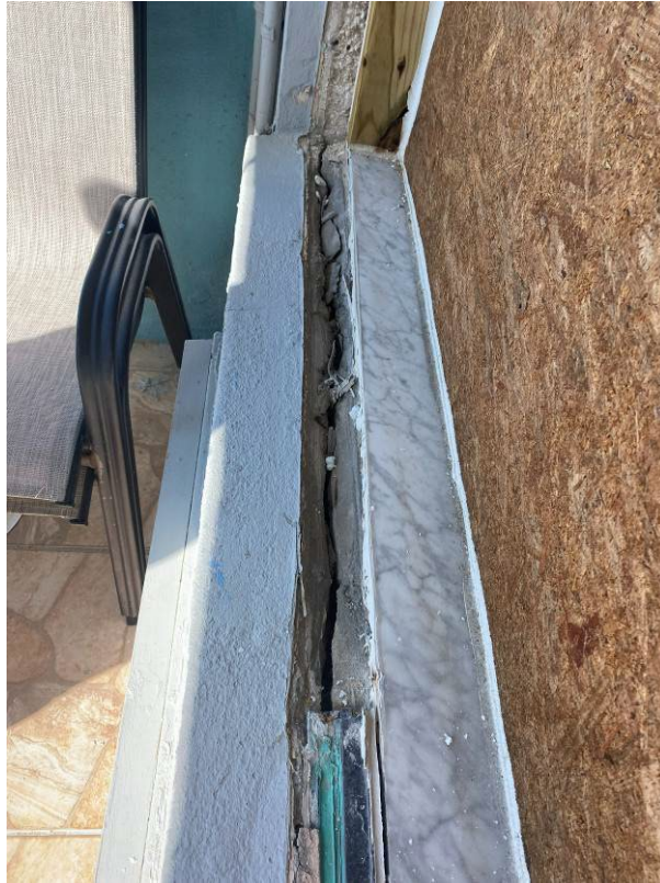
Photograph #21 – Window sill spalling with window removed
