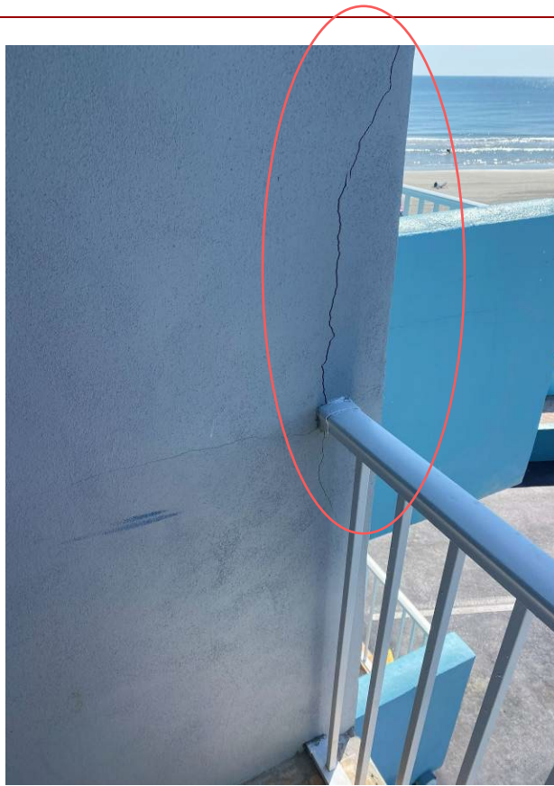
Photograph #19 – Typical wall spalling
