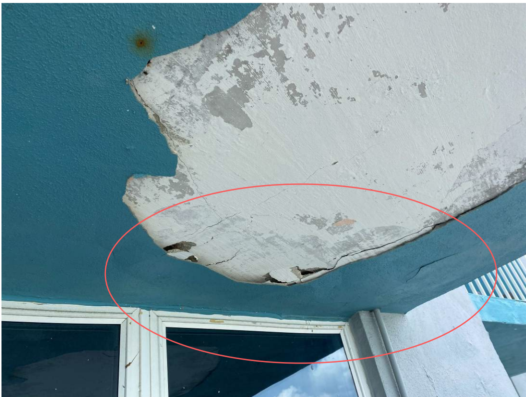
Photograph #12 – Typical ceiling spalling
