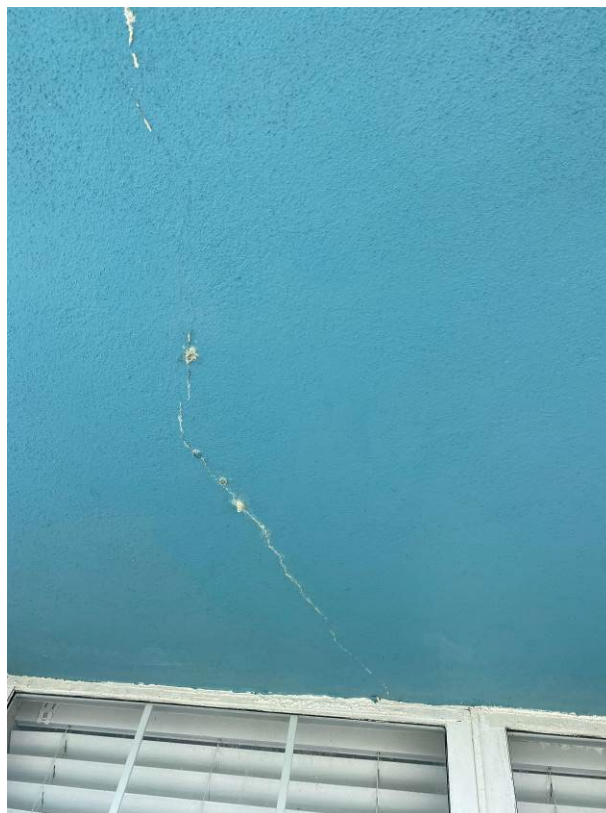
Photograph #10 – Typical concrete ceiling damage and stalactites
