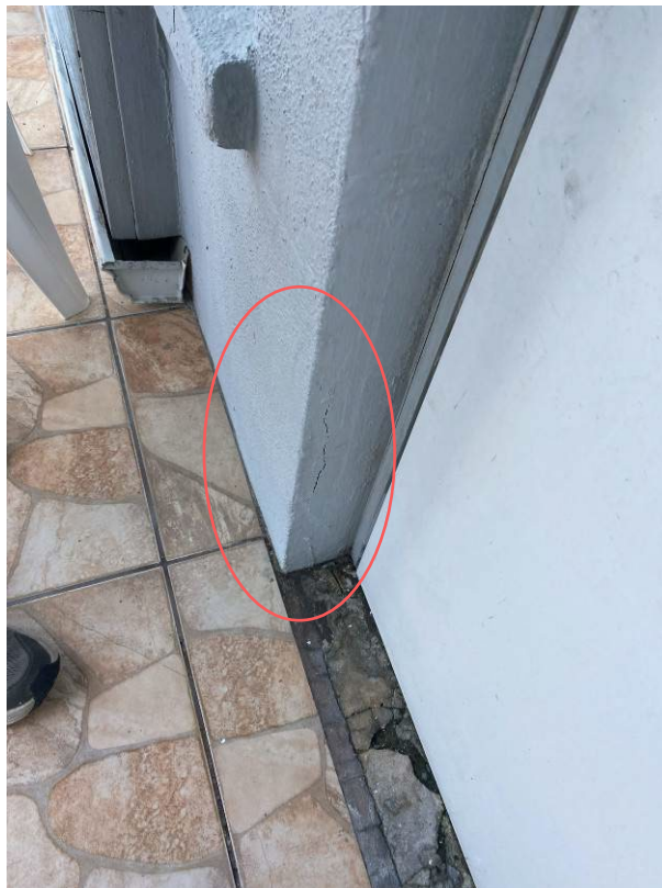
Photograph #16 – Typical wall spalling
