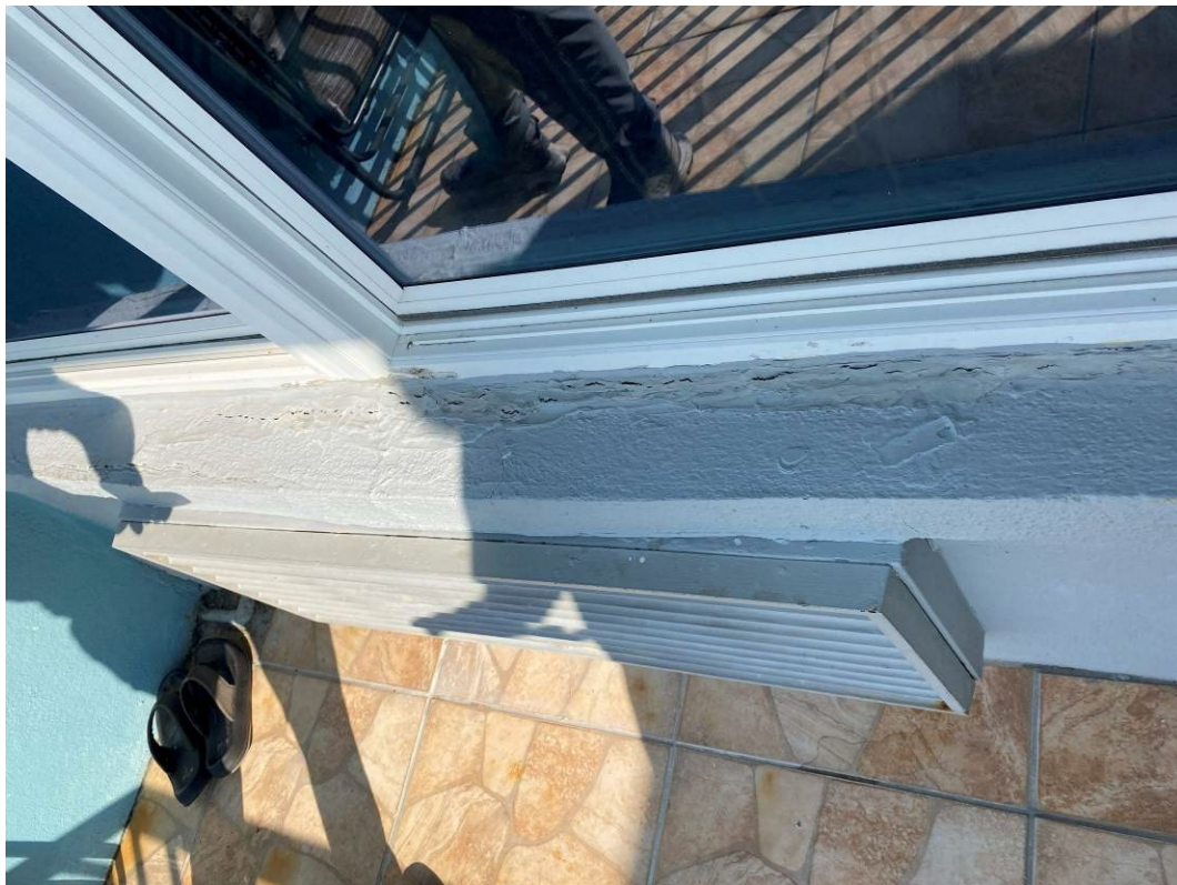
Photograph #4 – Typical window sill spall
