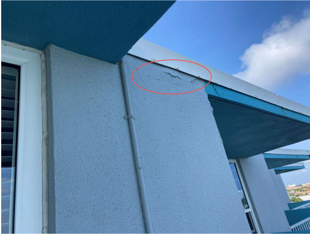
Photograph #3 – Typical concrete slab edge spall
