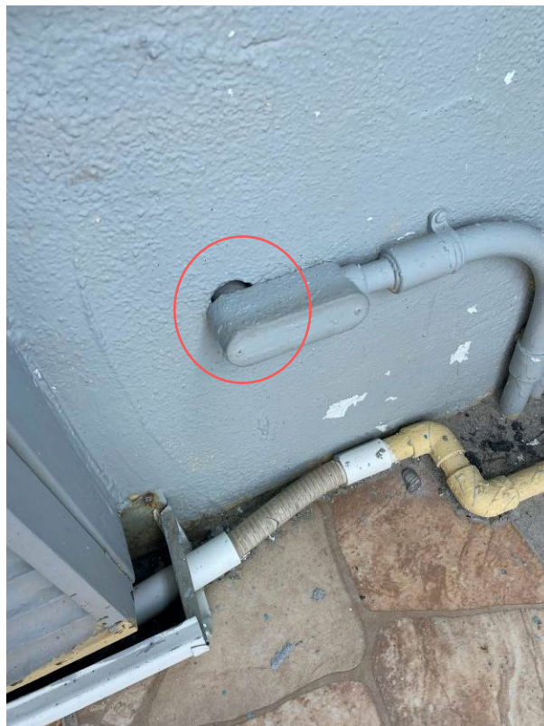
Photograph #28 – Typical unsealed hole at electric penetration
