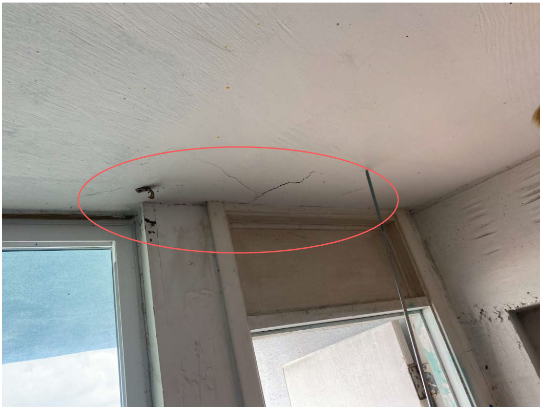
Photograph #14 – Typical interior ceiling concrete spalling
