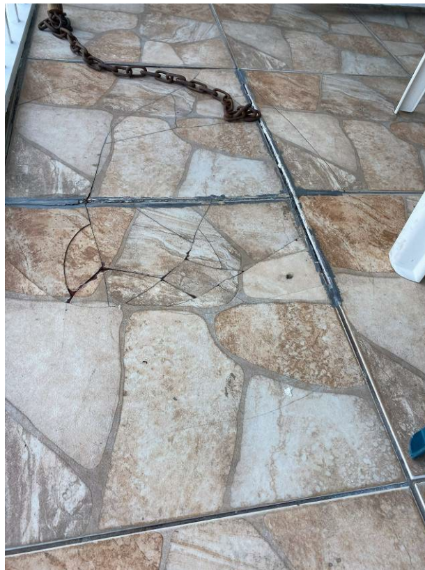
Photograph #24 – Typical tile cracking
