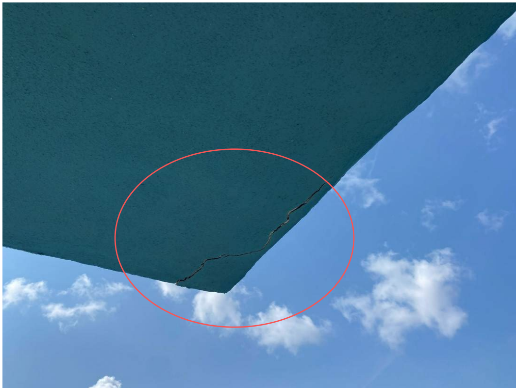
Photograph #8 – Typical slab edge spall
