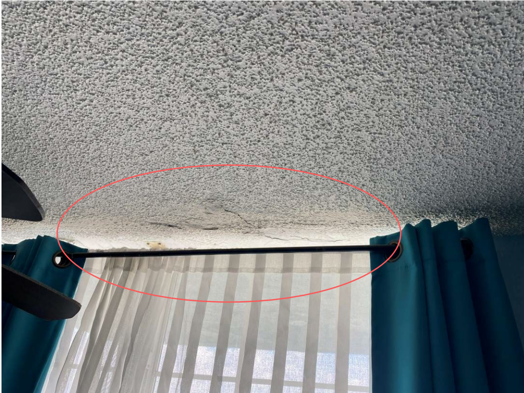
Photograph #9 – Typical interior ceiling spall
