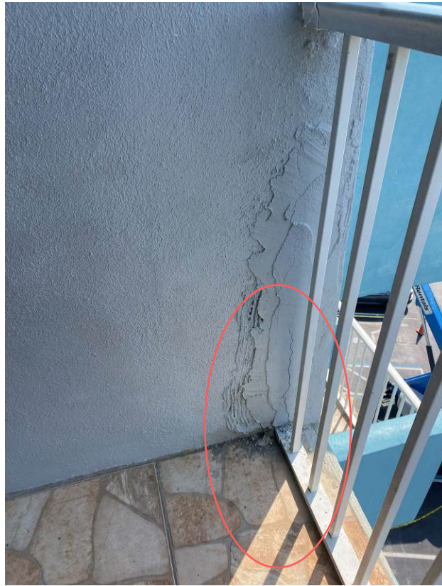
Photograph #5 – Typical concrete wall spall
