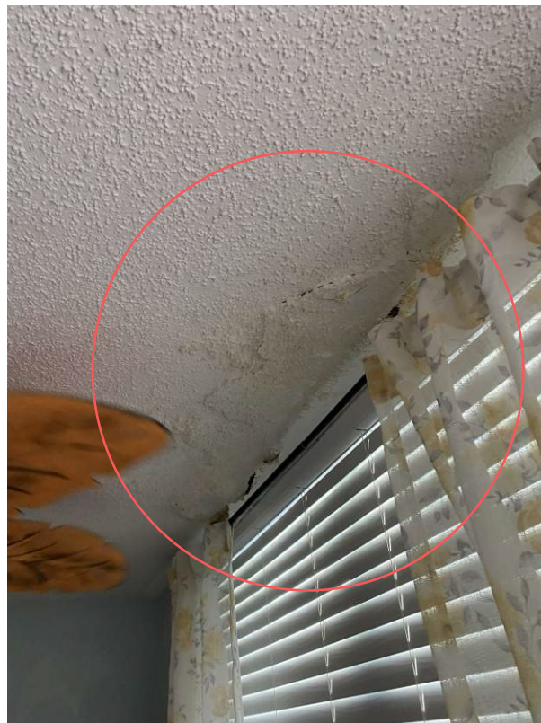
Photograph #22 – Typical interior ceiling spalling
