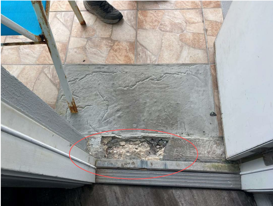
Photograph #11 – Typical topside concrete damage
