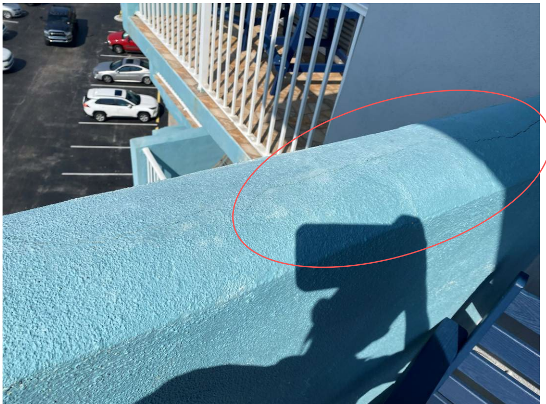
Photograph #6 – Typical guard wall concrete spall
