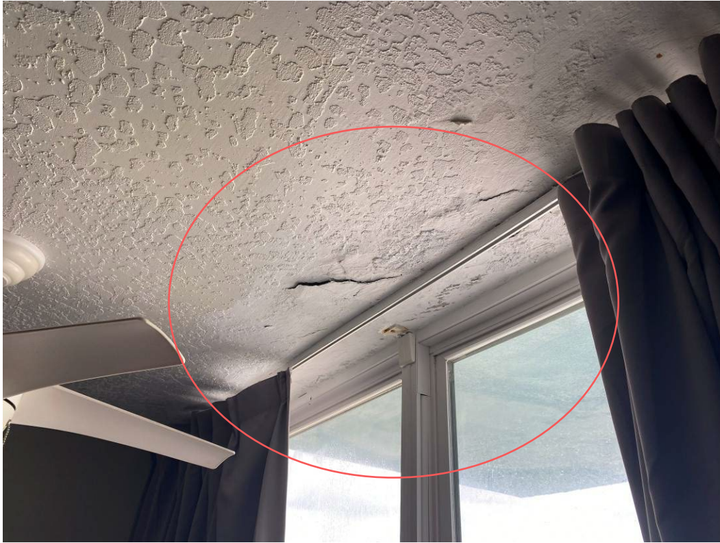
Photograph #15 – Typical interior ceiling concrete spalling
