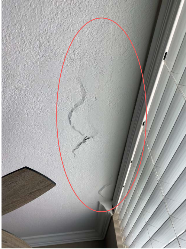
Photograph #17 – Typical interior ceiling concrete spalling
