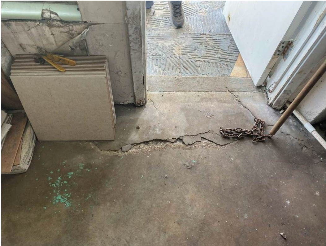
Photograph #1 – Typical interior topside concrete spall
