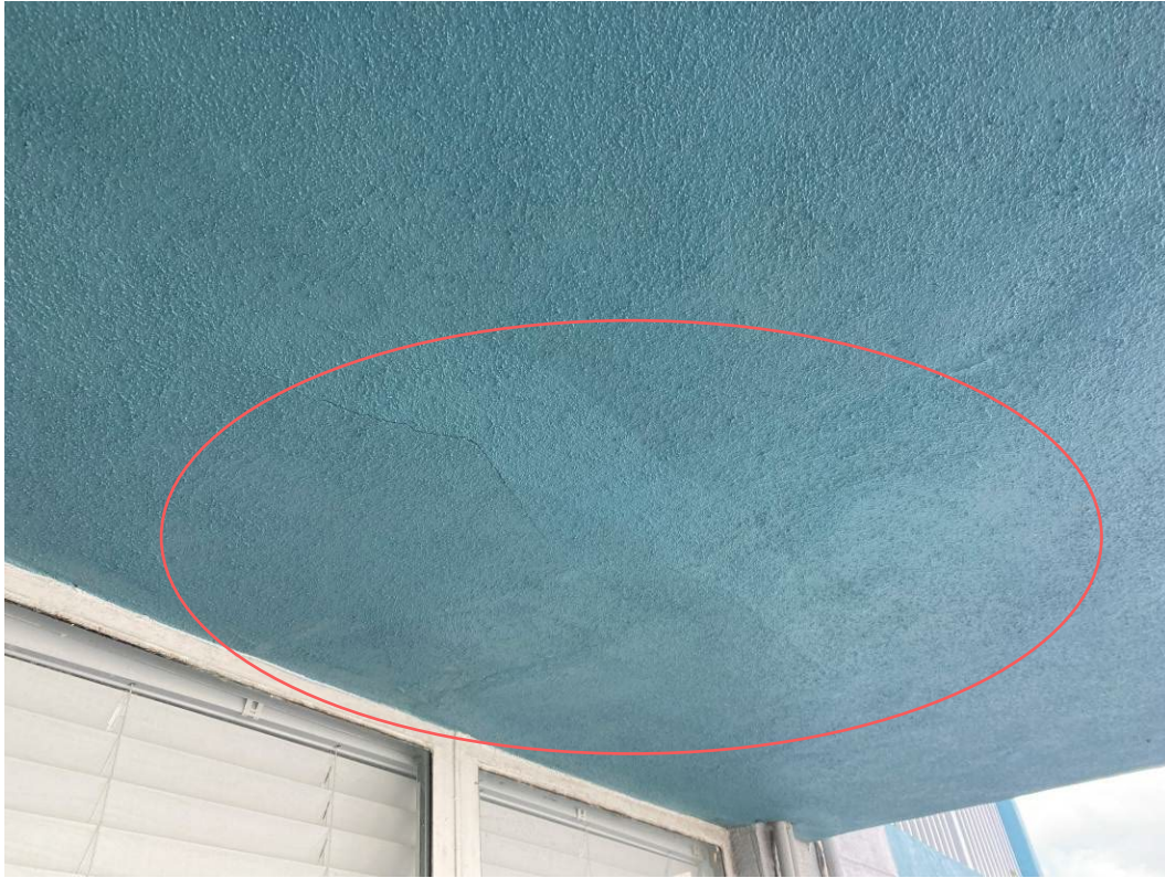
Photograph #23 – Typical ceiling spalling
