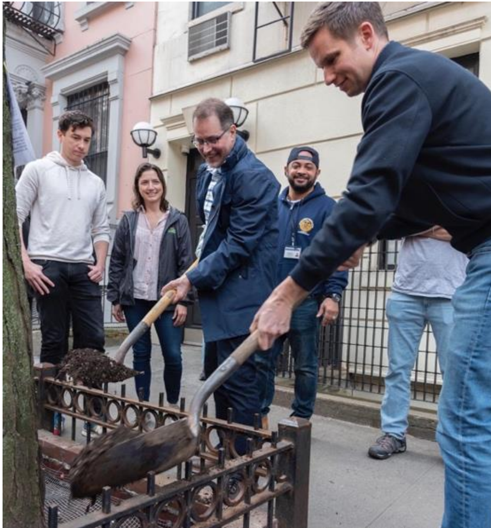
Backfilling a tree pit after installation of rat deterrent system by NYC Tree Pit Services. 03/18/22 Photo © Donna Rocco
