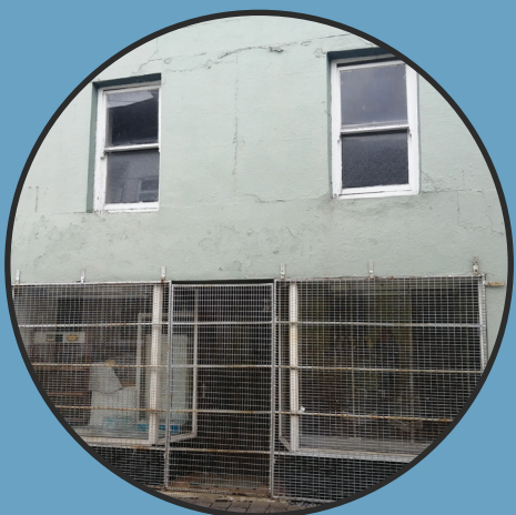
A derelict building in the town centre.
