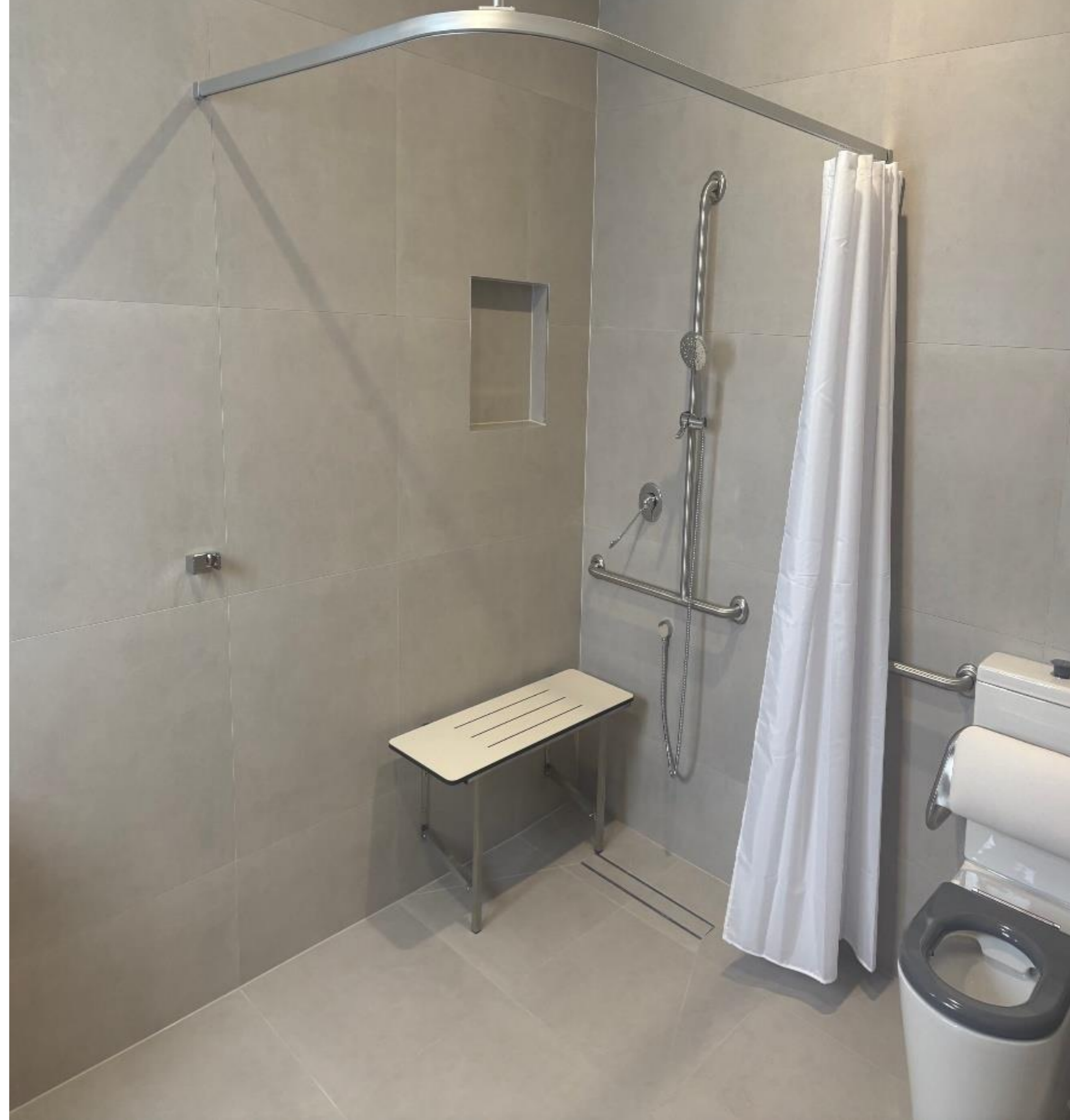
Image: Accessible bathroom with shower bench and grab rails. Supplied by Empowered Liveability, 16 April 2026.
