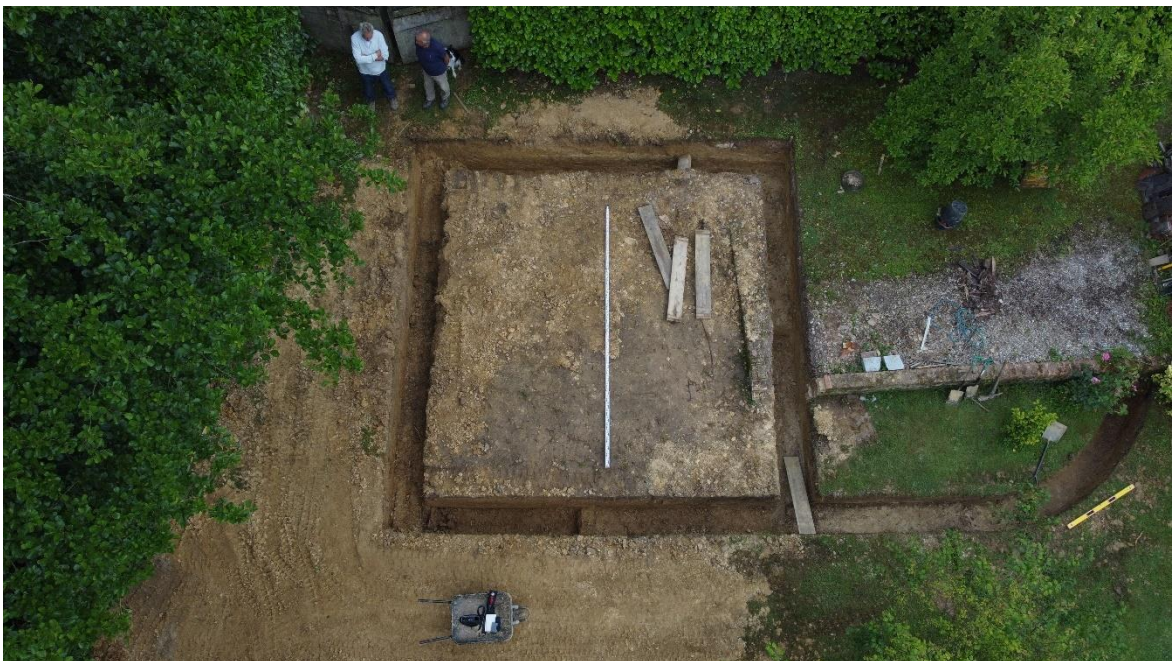
Plate 2 Aerial photograph of the development site following excavation of foundation trenches (4m scale)
