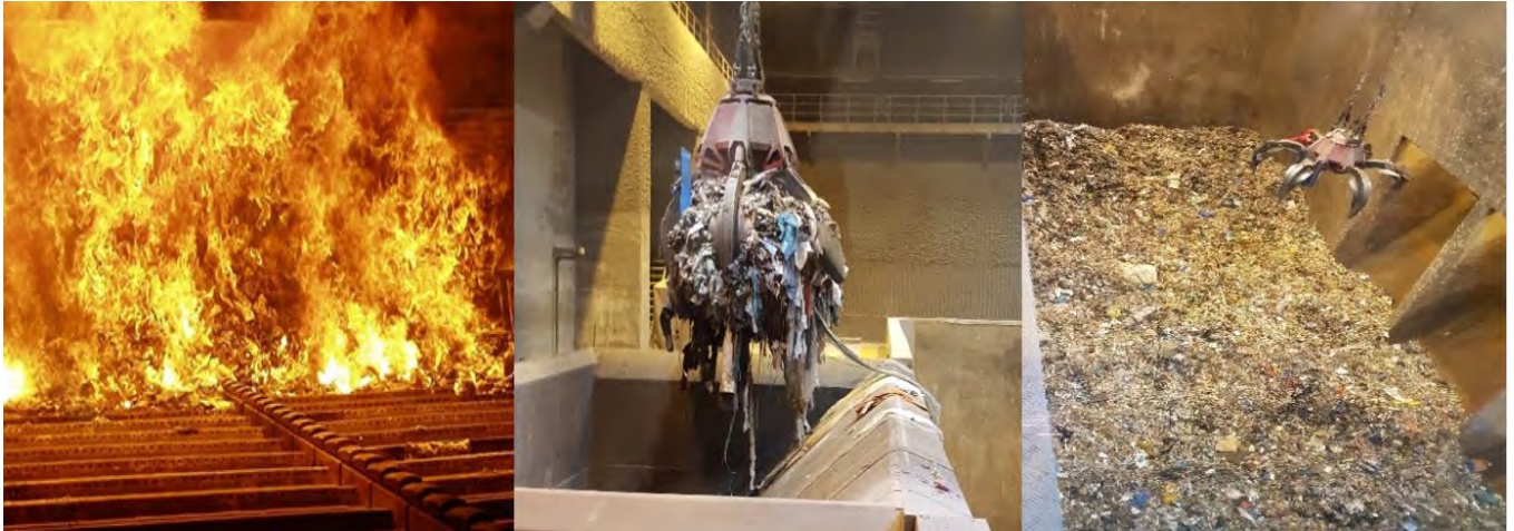
Figure 1 Waste burning at the grid. Waste transported to furnace (photo K. Bouman, 10-12-2019 REC)
