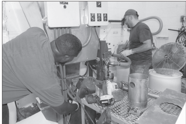
Brandon Waters, left, and Jose Ocegueda, 78th Civil Engineer Group water operators, make repairs to a soda ash feed system at a pump station at Robins Air Force Base Aug. 23. The soda ash systems are used to control water PH balance to the base water system. (U.S. Air Force photo by Joseph Mather)
