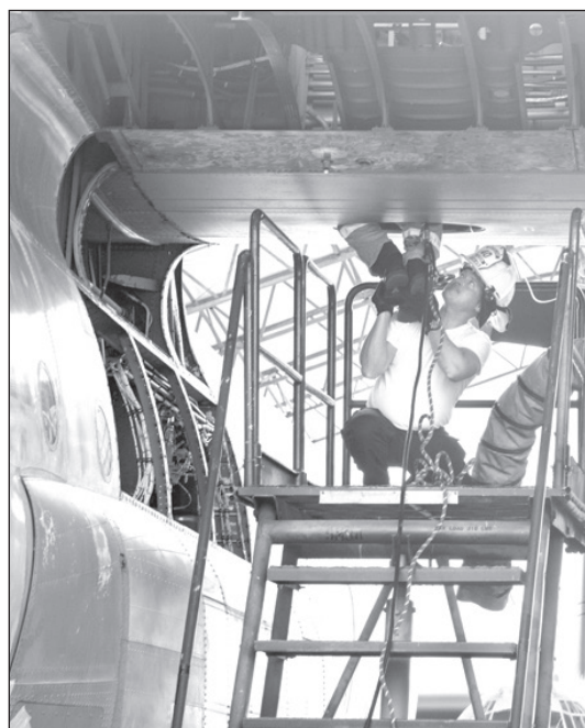
Fire Chief Jeffrey Kinzer, 778th Civil Engineer Squadron fire station chief, helps a firefighter into the wing cavity of a C-130J Super Hercules aircraft. Using a real aircraft allowed the fire and emergency services team to test their capabilities in a real-world environment. (U.S. Air Force photo by Patrick Sullivan)
