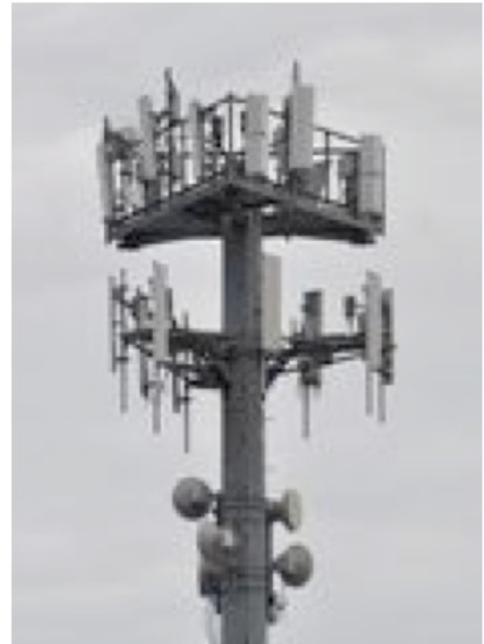
Traditional Monopole with multiple carriers in PROW
