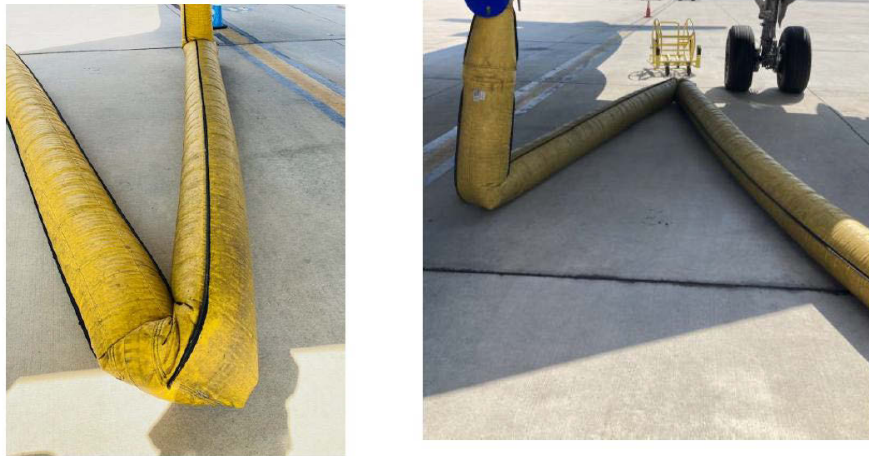
FIGURE 2-8 Examples of kinked hoses connecting preconditioned air units to aircraft. SOURCE: Scorsone (2025), used with permission from Air Line Pilots Association.
