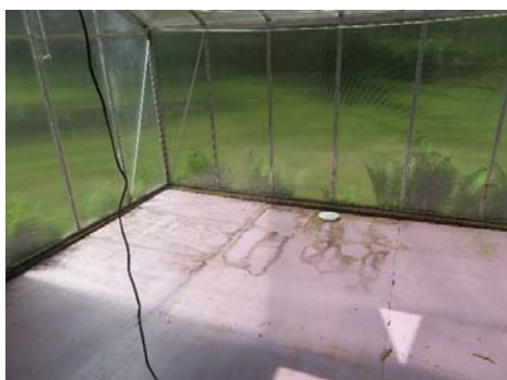
The old linoleum was taken up and as expected the wood was soaked. We (my husband & son) pulled up the plywood sheets, two layers, and set them up to try to dry. This took all week because it was raining outside for a few days.
