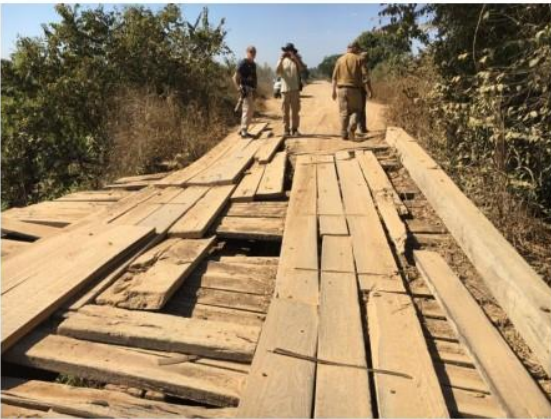
Broken down bridge along the Transpantaneira "highway"
