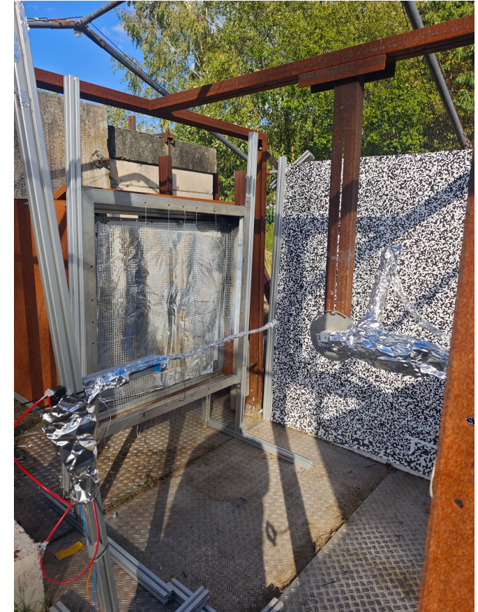
Free field test site of ITES-KIT with installed experimental rig for impingement (images courtesy of KIT)
