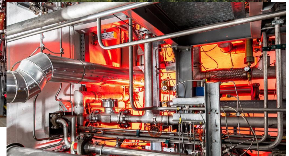
High pressure cryogenic lines
