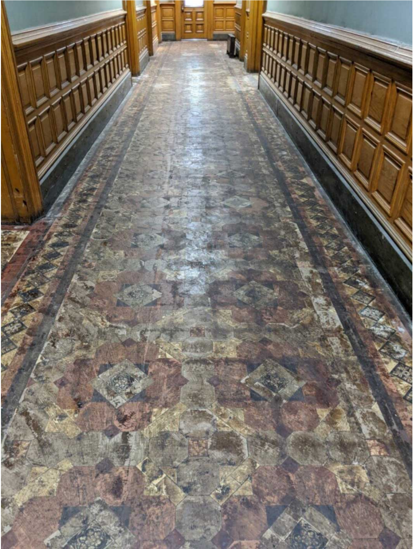
Original Stoke-on-Trent tiles dating to the mid-1800s were buried beneath vinyl flooring that was installed in the 1960s. Photo via @StevenFulop/Instagram.
