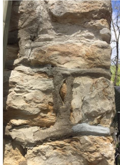
The upper most mortar in this image is the proper limestone mix. Note its white-ish color. Also note the improper concrete
