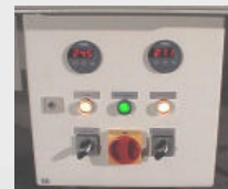
Central switchbox with precise electronic controller
